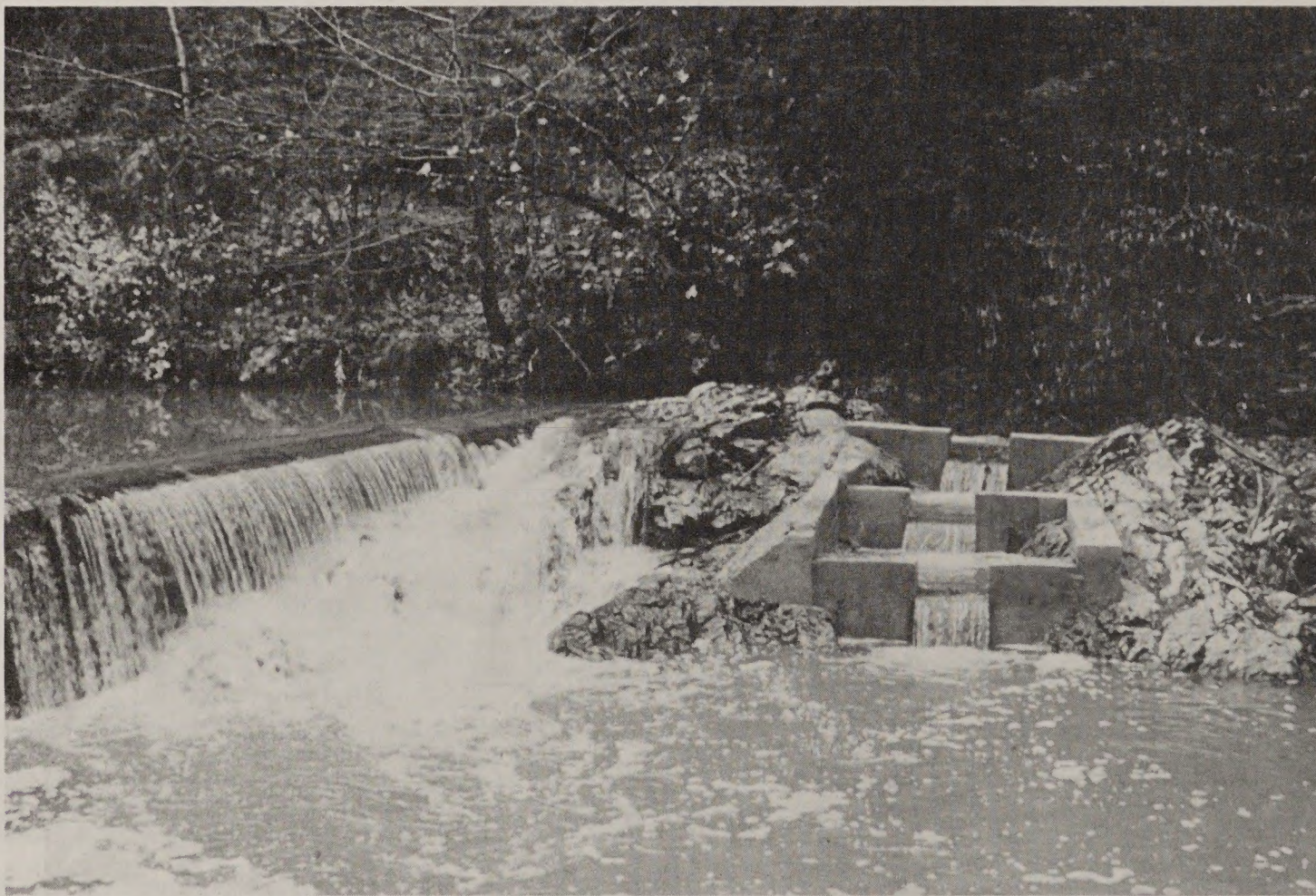
9. This concrete step-and-pool fishway was constructed at a low irrigation dam to provide anadromous fish easy access to upstream spawning areas at all streamflows.
