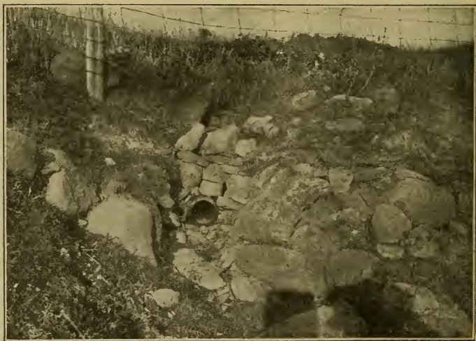
PLATE IX. DRAINAGE. — The drain outlet is often poorly constructed and easily clogged, as shown in the upper figure. The lower one is well protected.
