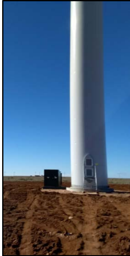
Figure 8. Typical pad-mounted transformer.
