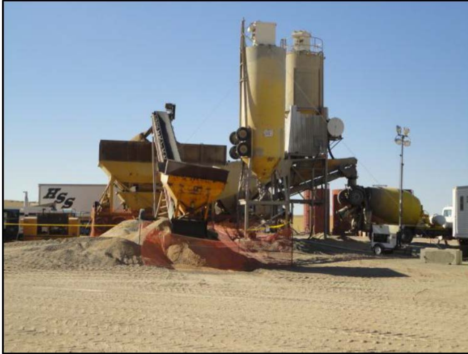
Figure 18. Typical temporary concrete batch plant.
