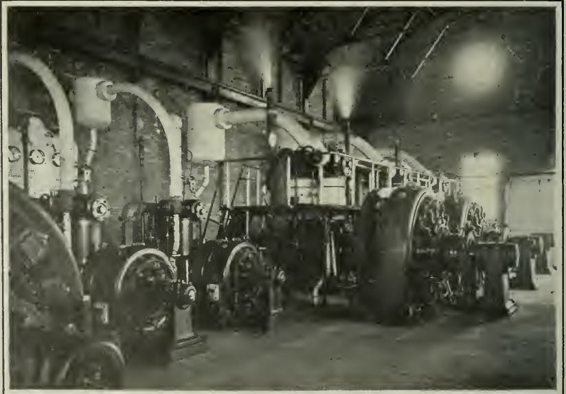
FRUITPORT POWER HOUSE, G. R., G. H. & M. RY. FIVE 250-KILOWATT WESTINGHOUSE GENERATORS.
