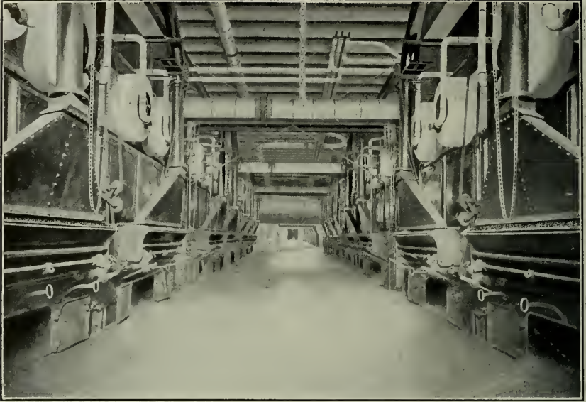
RONEY MECHANICAL STOKERS, 96TH STREET POWER HOUSE, METROPOLITAN TRACTION CO., N. Y.
