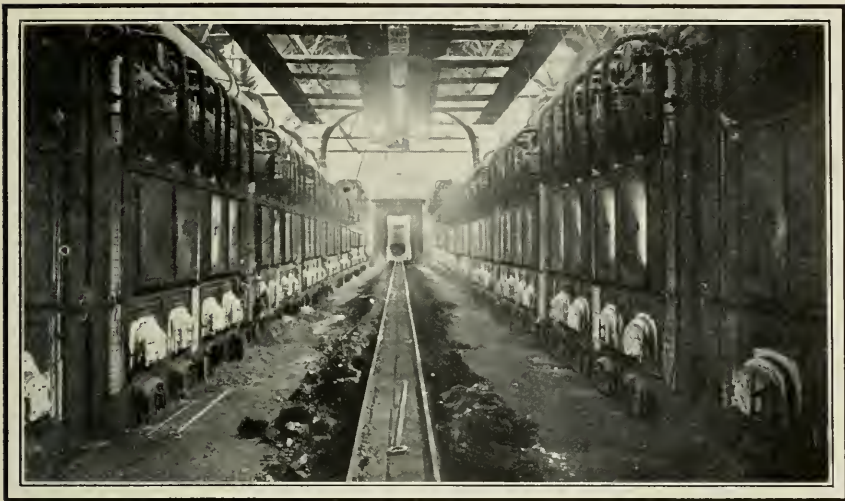
A 25,000-HORSE-POWER BOILER PLANT.
