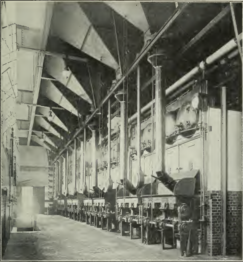
VICARS' STOKERS IN A LARGE LONDON POWER STATION.
