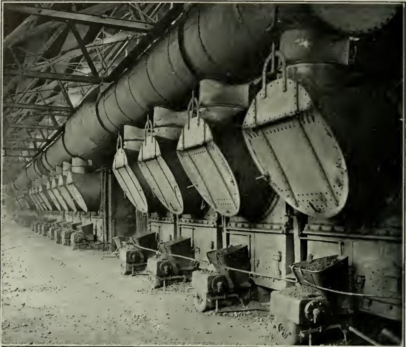
AMERICAN STOKERS, UNDERFEED SYSTEM, AT THE HOMESTEAD MILLS, CARNEGIE STEEL CO., UNITED STATES STEEL CORPORATION, PITTSBURG, PA.
