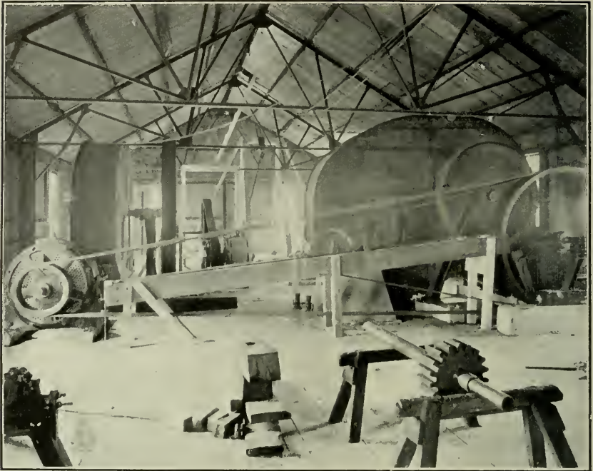
INDEPENDENT ELECTRIC MOTORS DRIVING SUCTION FANS.
