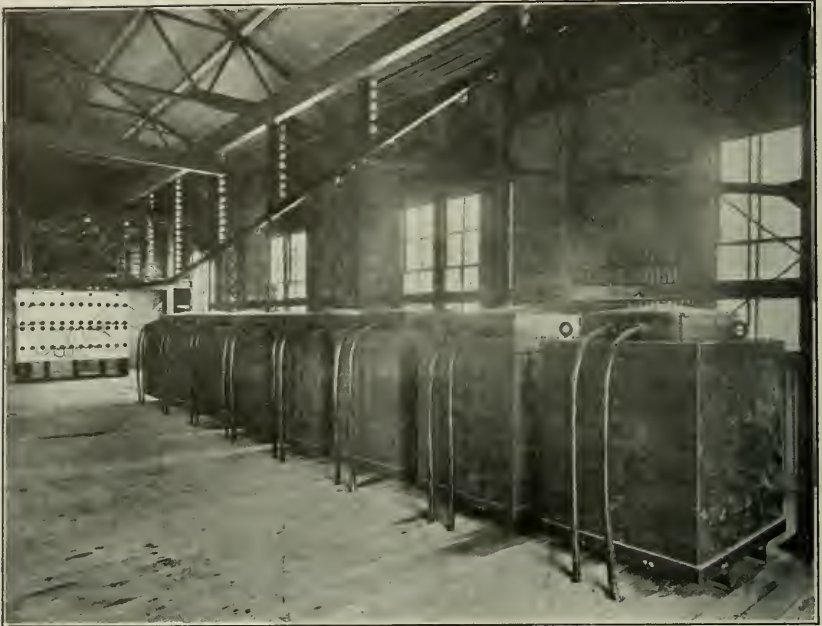
HIGH POTENTIAL TRANSFORMERS, HELENA, MONTANA..
