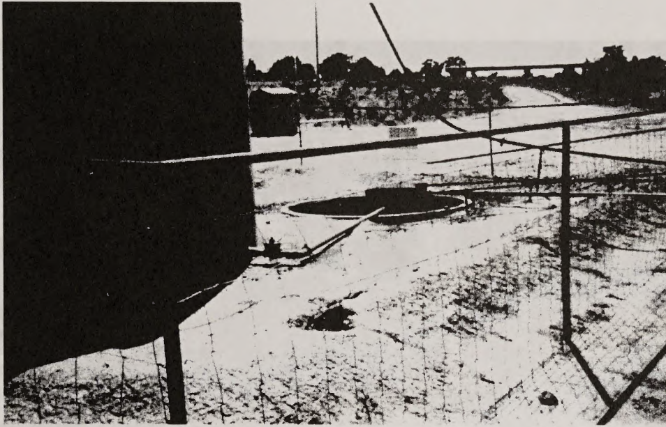
Photo 3-7 Typical Condensate Tank and Produced Water Pit (only associated with conventional wells)
