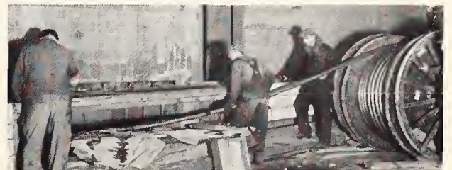
Above—Copper cable being unreeled and installed in the new tunnel. Enough cable, conduit and wire was installed to reach from New York City to Omaha, Neb. Complete control over traffic, lighting and ventilation is assured at all times and there are two emergency power sources, if they are ever needed . . . .
