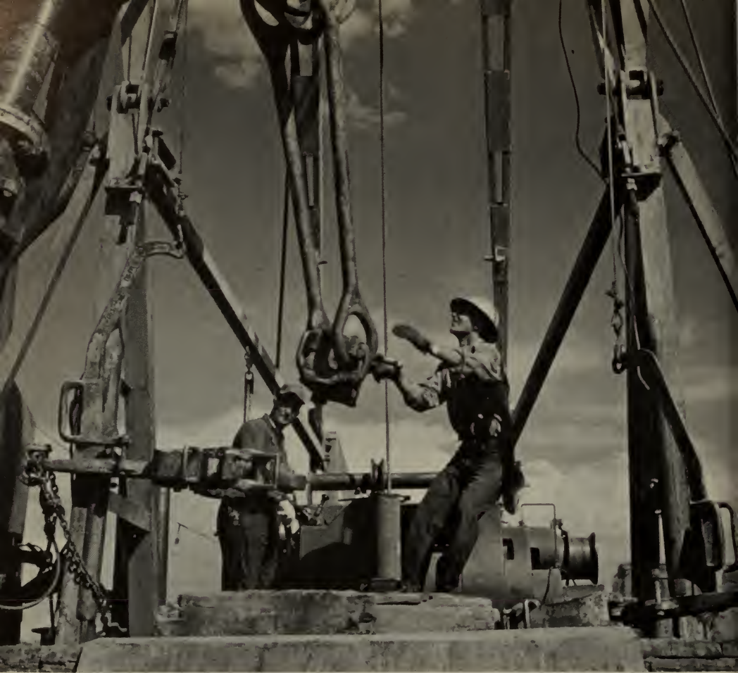
Pulling a core barrel during exploration for potash on public lands at Cane Creek, Utah. This work led to discoveries resulting in a new industry for Utah with an initial investment of $25 million for new access roads, plant, mineshaft, railroad, etc.
