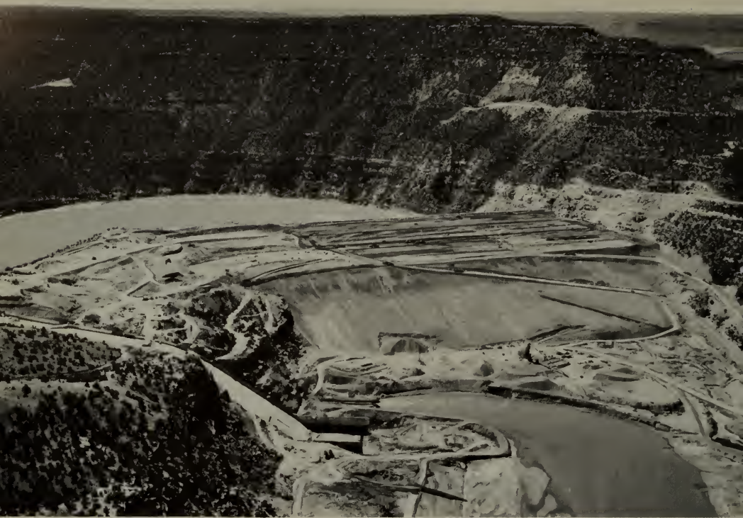
Men and machines place and compact earth in Navajo Dam on the San Juan River in New Mexico.
