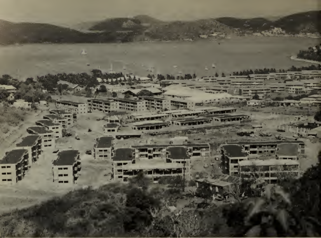
View of the Oswald E. Harris Court, a 300-family public housing project under construction in St. Thomas, Virgin Islands. It is expected that this project will be completed by January 1962. It will help to relieve the extreme shortage of adequate housing in St. Thomas.
