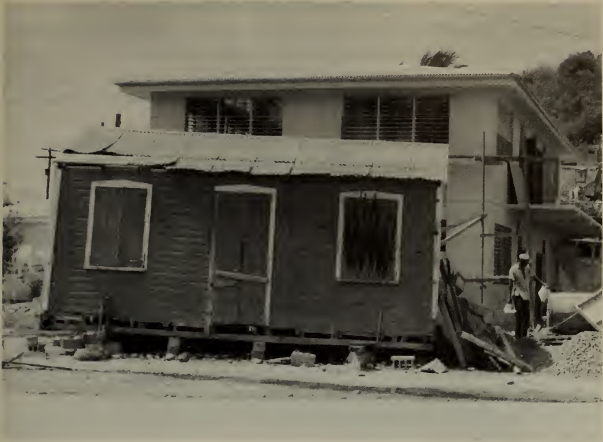
New Kindergarten School at French Village, St. Thomas, Virgin Islands, under construction. The wooden building in the foreground was formerly used as a kindergarten school.
