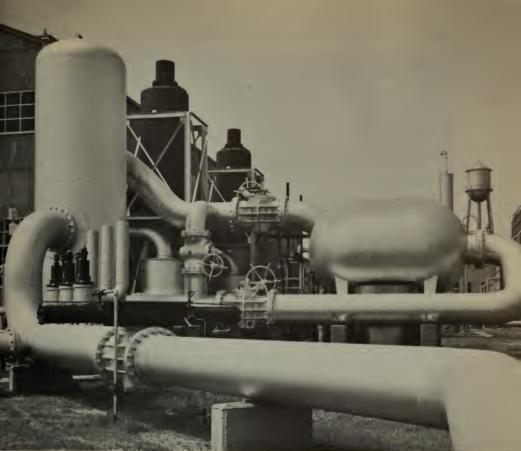
This gas-cleaning equipment was added to the Bureau's Exell, Tex., plant during the year to increase its processing capacity to 130 million cubic feet per day.
