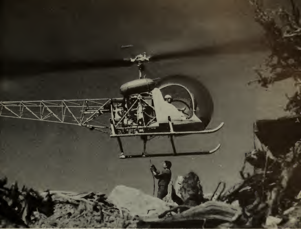
A lineman attaches the lead or "soek" line to helicopter for a 2,000 foot run to bridge a deep, precipitous canyon with Bonneville Power Administration's Rocky Reach-Maple Valley 345,000 volt transmission line.
