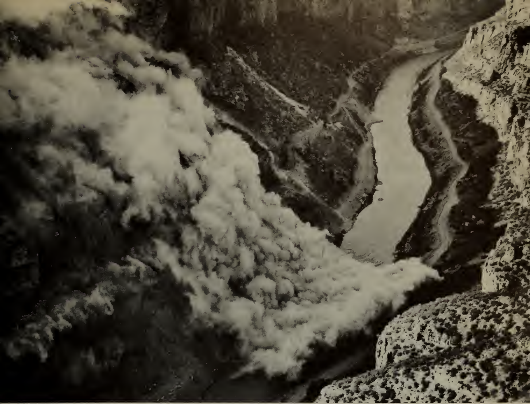
A dynamite blast launches preliminary construction on Yellowtail Dam on the Big Horn River in Montana.
