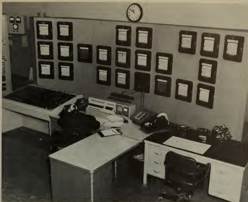
Springfield dispatcher's office, Springfield, Mo., is the nerve center of SPA's electric transmission system in Missouri and Arkansas. Information regarding the power flow between the SPA system and other systems is telemetered into this office for use in automatic load control equipment.
