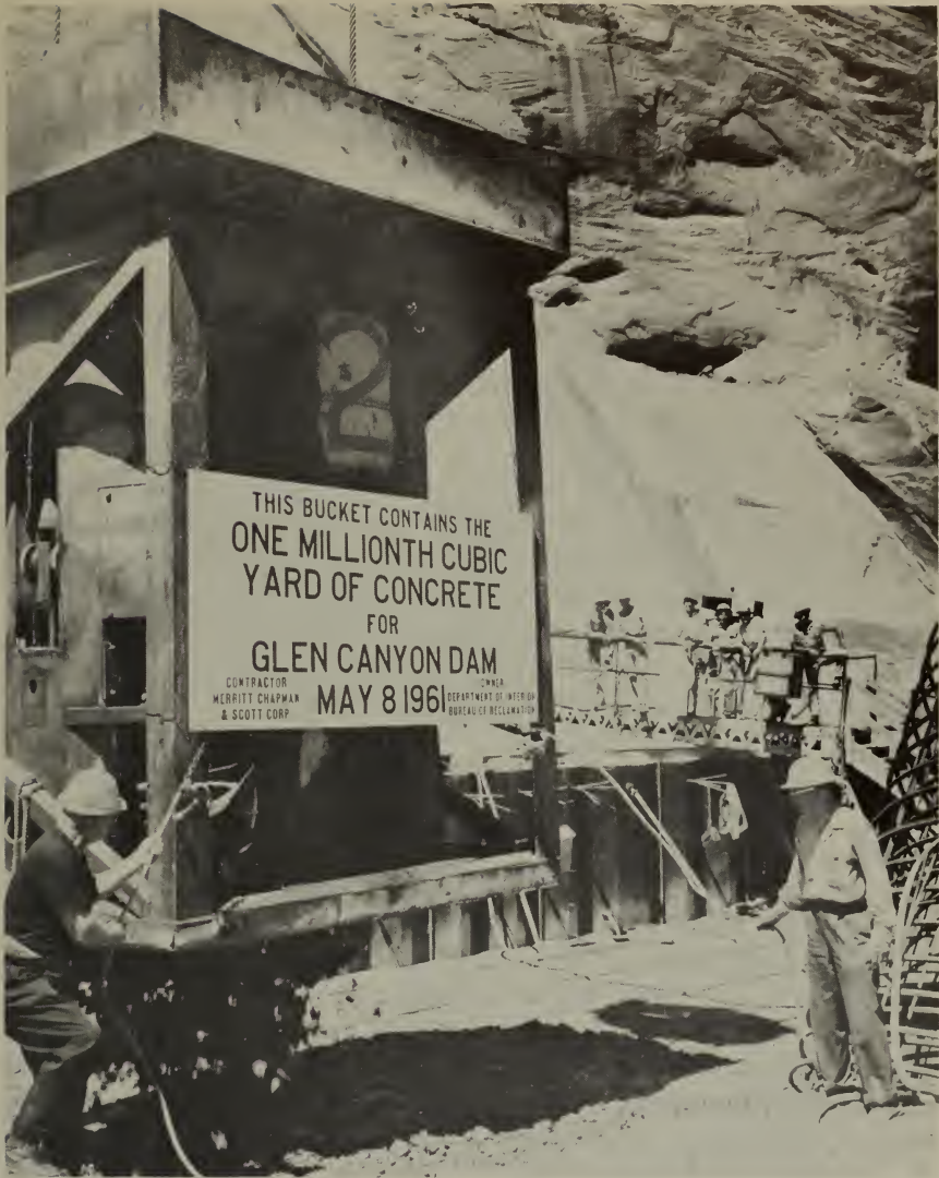
Engineers pull lanyard releasing 1-millionth cubic yard of concrete into Glen Canyon Dam.
