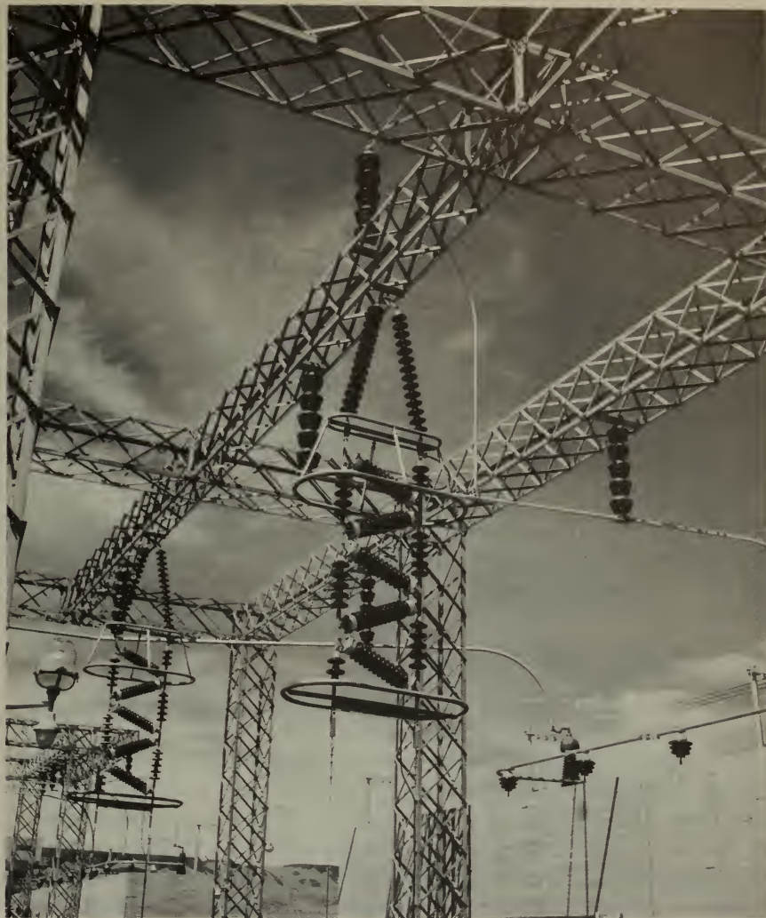
Suspended 230,000 volt lightning arresters form an intricate pattern atop the McNary Dam powerhouse.
