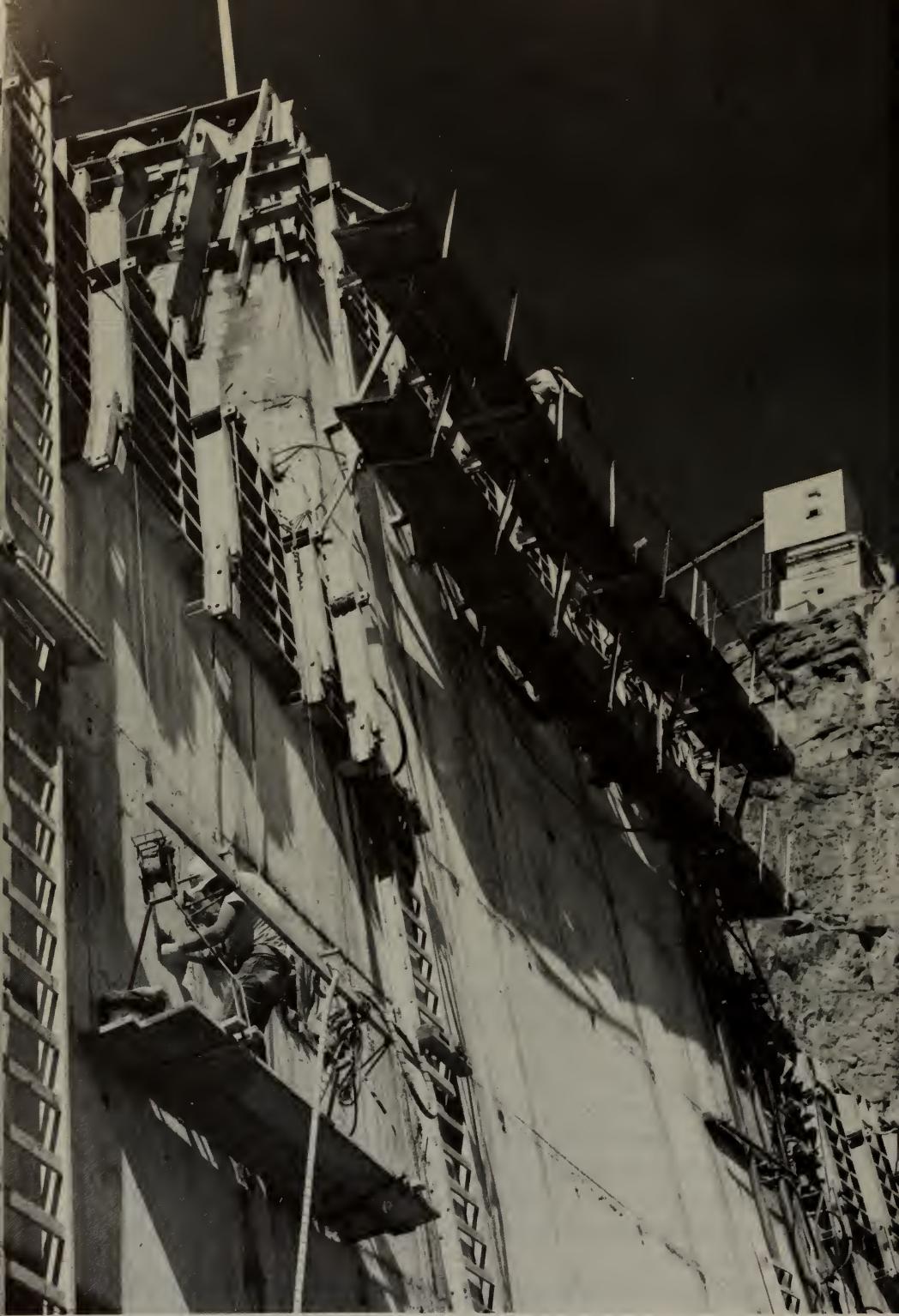
Men work on concrete face of Flaming Gorge Dam on Green River in Utah as structure rises toward its ultimate height of 502 feet.
