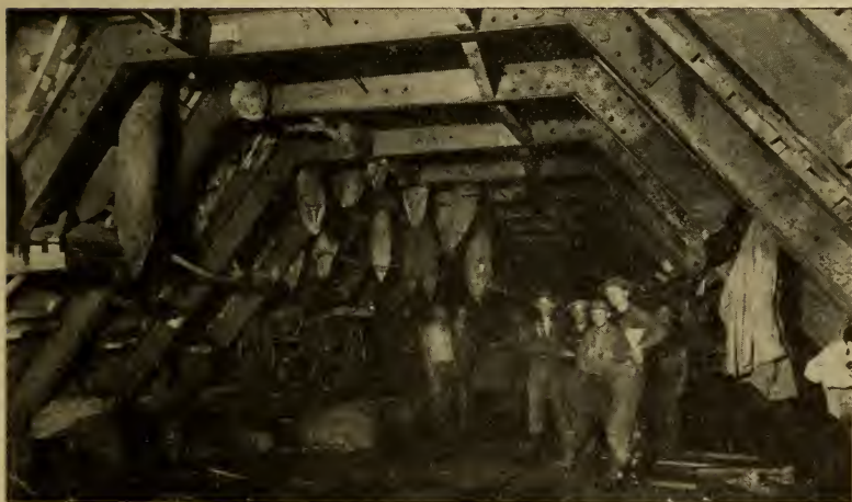
FIG. 110. Steel I-beam sets for roof timbering. American system. Hudson & Manhattan Railroad, Jersey City, N. J.
