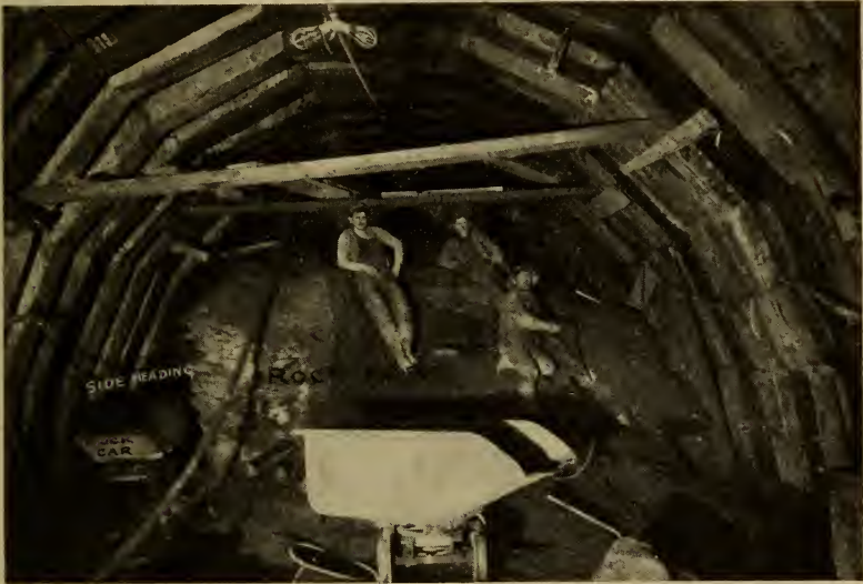
FIG. 107. American system of excavating and timbering. Hudson & Manhattan Railroad, Jersey City, N. J.
