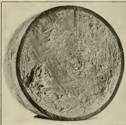
Delivery Pipe from Injector Completely Filled with Scale
