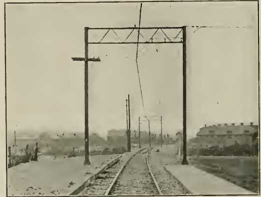
View of Overhead and Feeder
