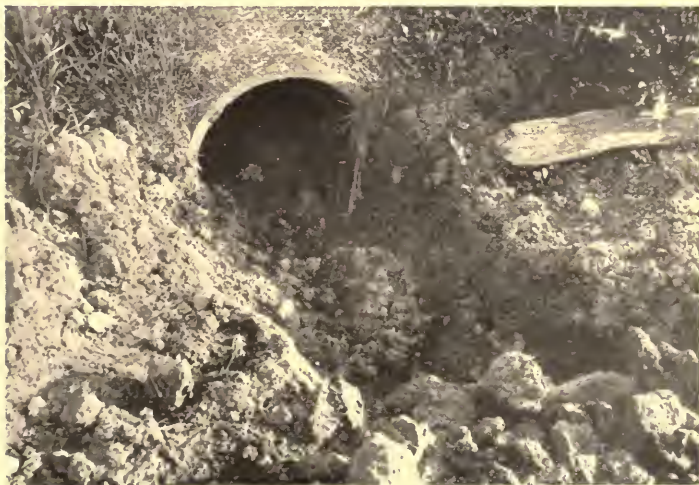
77. OUTLET OF A TILE DRAIN CLOGGED BY SOIL SO THAT THE DRAIN DOES NOT WORK
