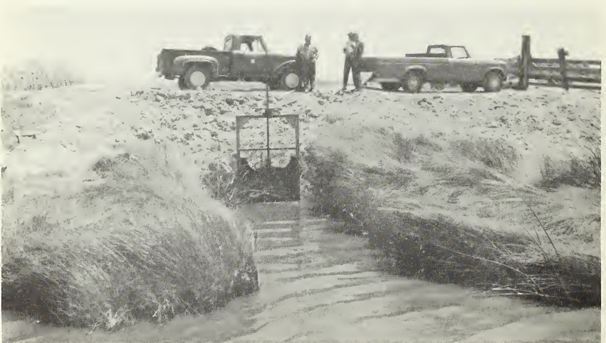
Photo 7. Above type of water control structure installed.
