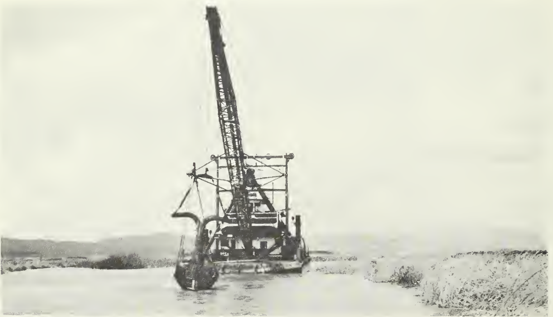
Photo 5. Floating dredge used for constructing and repairing exterior levees and cleaning tidal inlets and outlets at water control structures.
