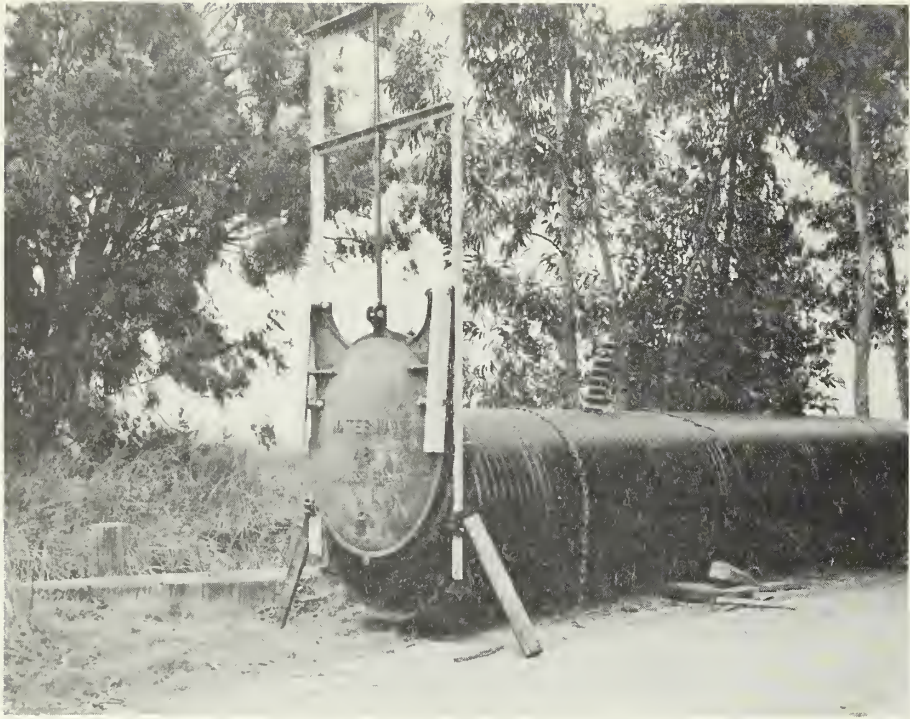
Photo 6. Asphalt coated corrugated metal pipe with attached combination slide and flap gate used as tidal water control structure.
