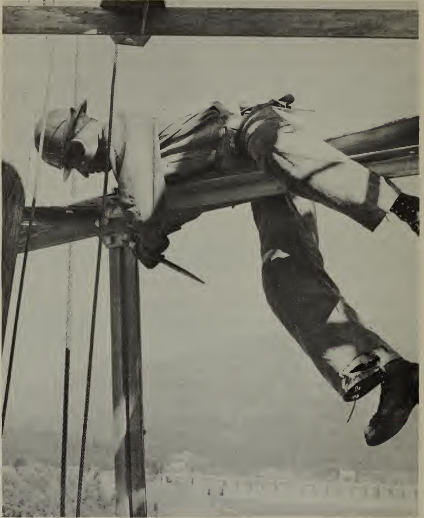
A construction worker erects a steel tower on one of BPA's high voltage transmission lines against a background of the Bonneville Dam spillway.
