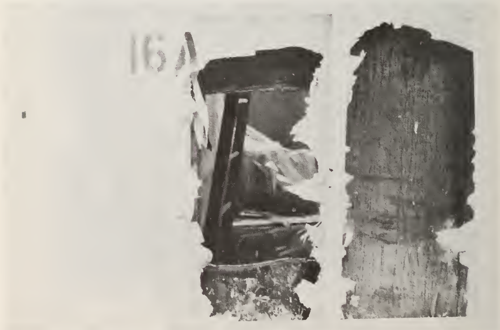
Figure 149. Test 16A. Final Opening
