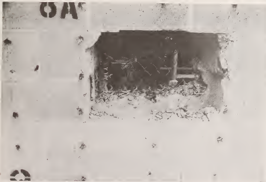
Figure 63. Opening Produced in Test 8A
