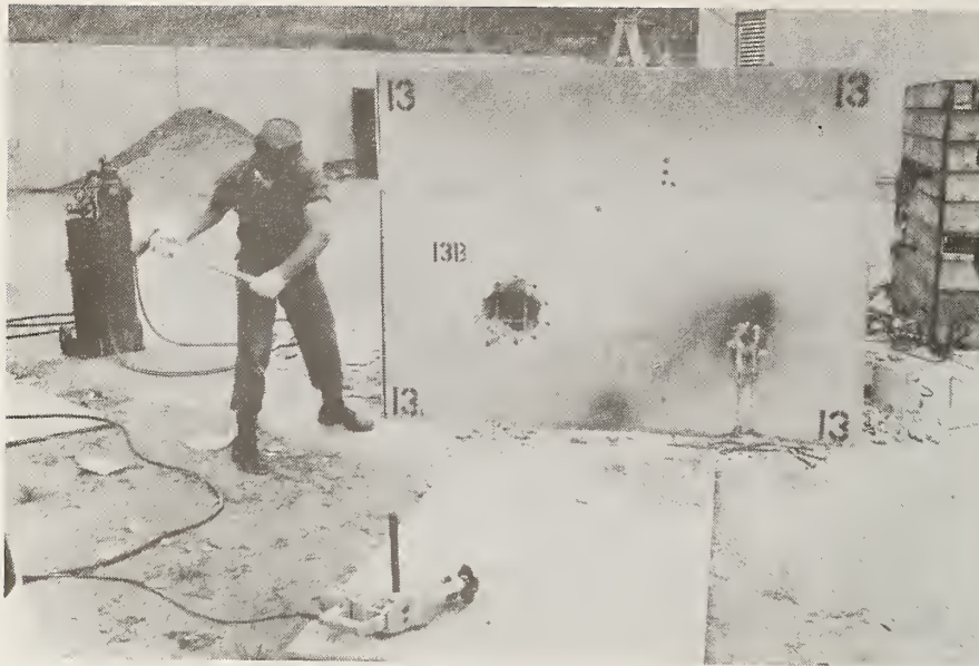
Figure 113. Test 13B Using Taper Punch to Spall from Edge of Holes into Central Opening
