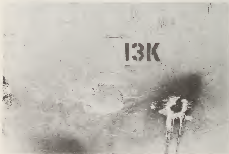
Figure 124. Spalling Produced by 301 Blows from Battering Ram ; Test 13K 100
