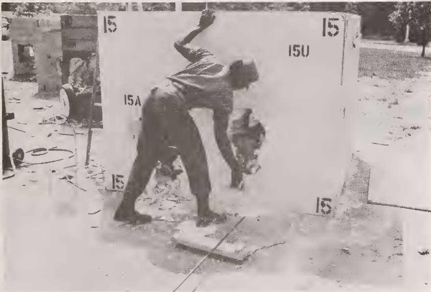
Figure 140. Test 15U. Opening Produced by Kicking Out Plasterboard
