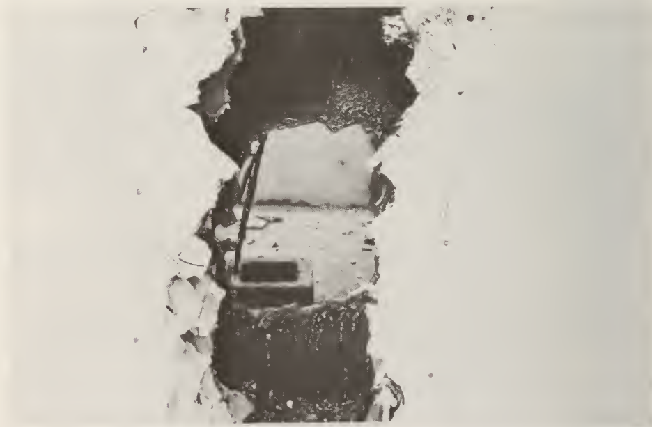
Figure 151. Hole Produced by Burning Bar; Test 16U
