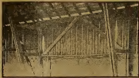
The trusses are placed 15 feet apart; 2x12's are the heaviest timbers used
