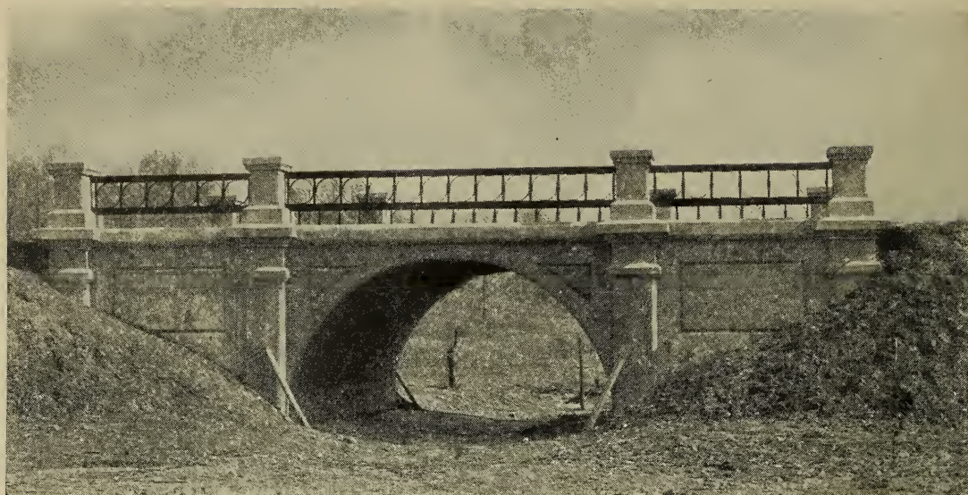
83. The combination of an iron railing with this concrete structure possibly saved money—but some day the railing must be replaced.
