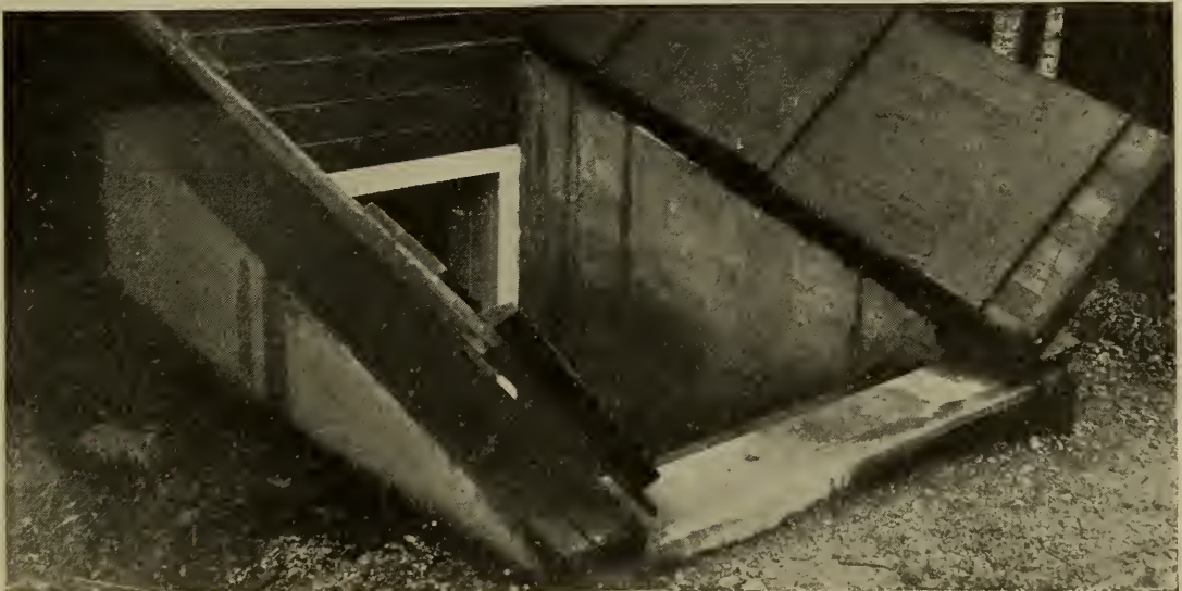
12. A later view of the cellarway shown under construction on the opposite page. The bolts which hold the hinges of the door were placed in the fresh concrete.
