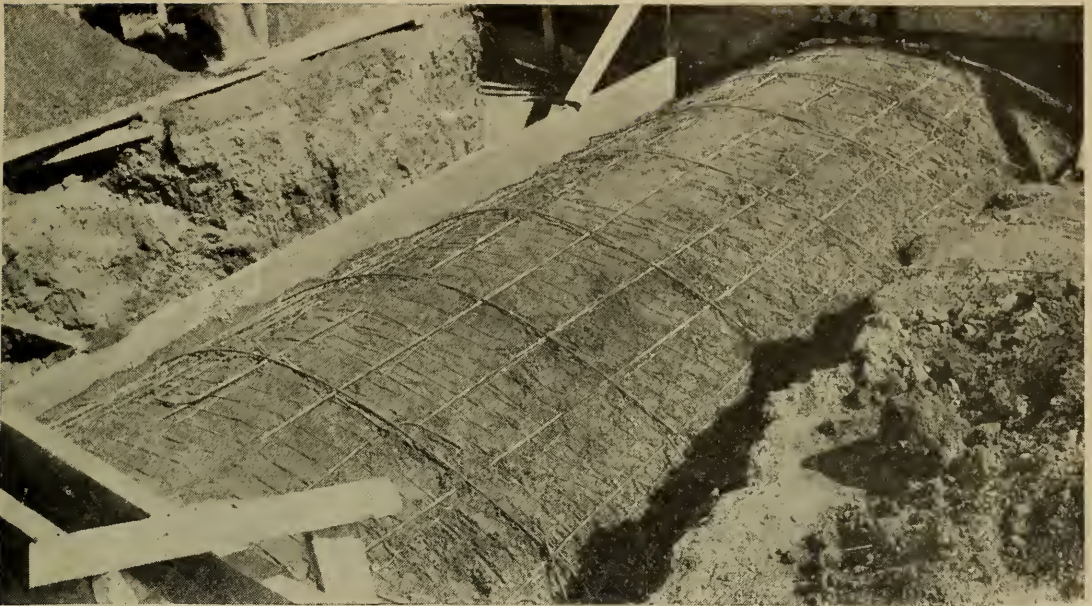
81. Method of placing reinforcing in small culvert or bridge, showing lateral and longitudinal reinforcing. Spacing and size depend on size of structure.
