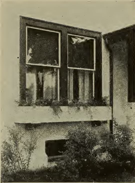
21. This concrete window-box was built in as the sill for the double window.
