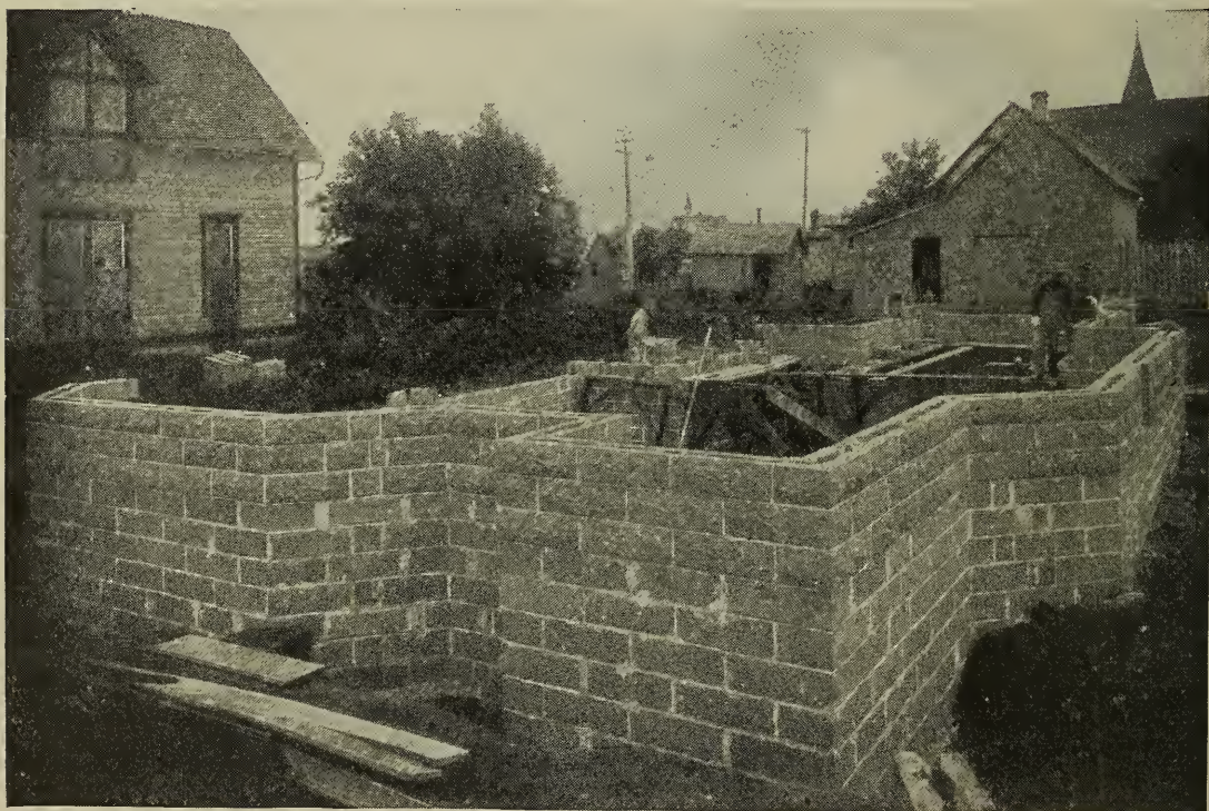
5. Concrete block foundation, laid in cement mortar. The hollow blocks give a non-continuous air space.
