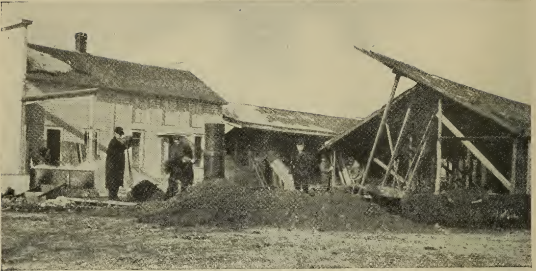
4. Heating of materials in cold weather. The aggregates are so placed as to be easily shoveled next to the heater.
