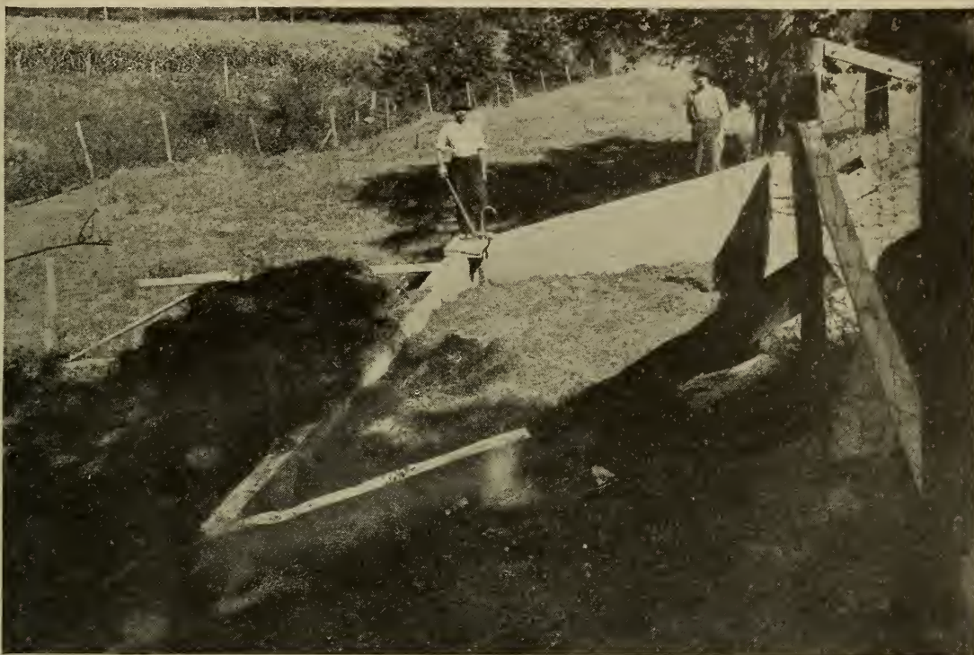
59. Concrete manure pit, showing sump well in far corner. Construction plan for such a pit is shown on next page.
