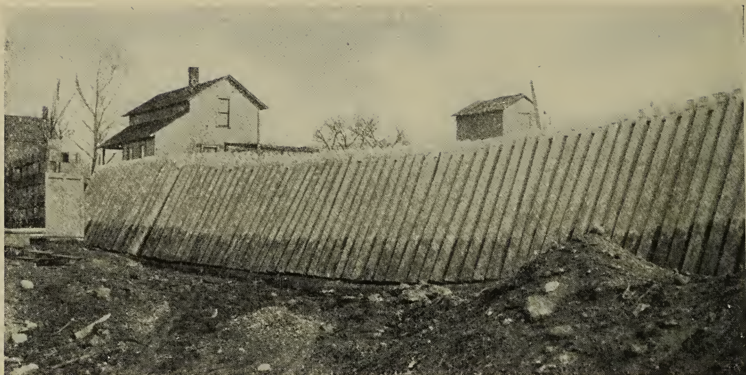
29. Concrete posts and rails curing for use in fence similar to that at foot of page. The time of curing in this case averaged two months.
