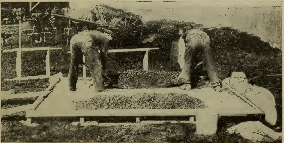
2. Process of shoveling sand and stone in hand mixing. The ideal method is with each man shoveling half way but spreading the full distance of the board.
