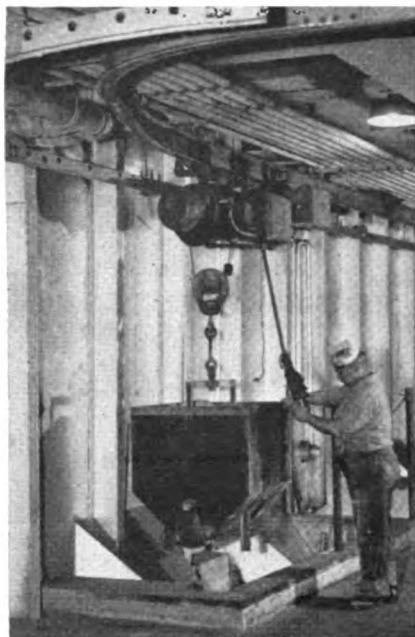
A completely enclosed sand bin and exhaust system help keep the silica count within permissible limits.
