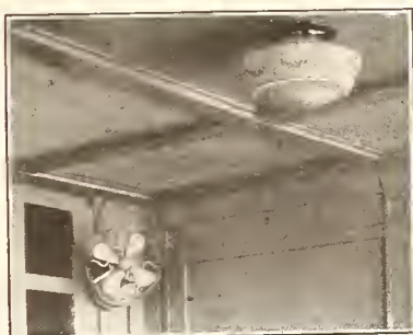
Efficiently equipped Demonstrating Room, showing Unico Lighting and Ventilating Units Installed. Comfort to your customer brings greater record sales.
