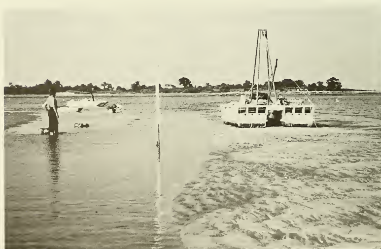
Figure 7. Barge on the Crest of a Sand Wave. Long staff in center is a tide gauge. The pipe to the right of the gauge is part of the diver support system.
