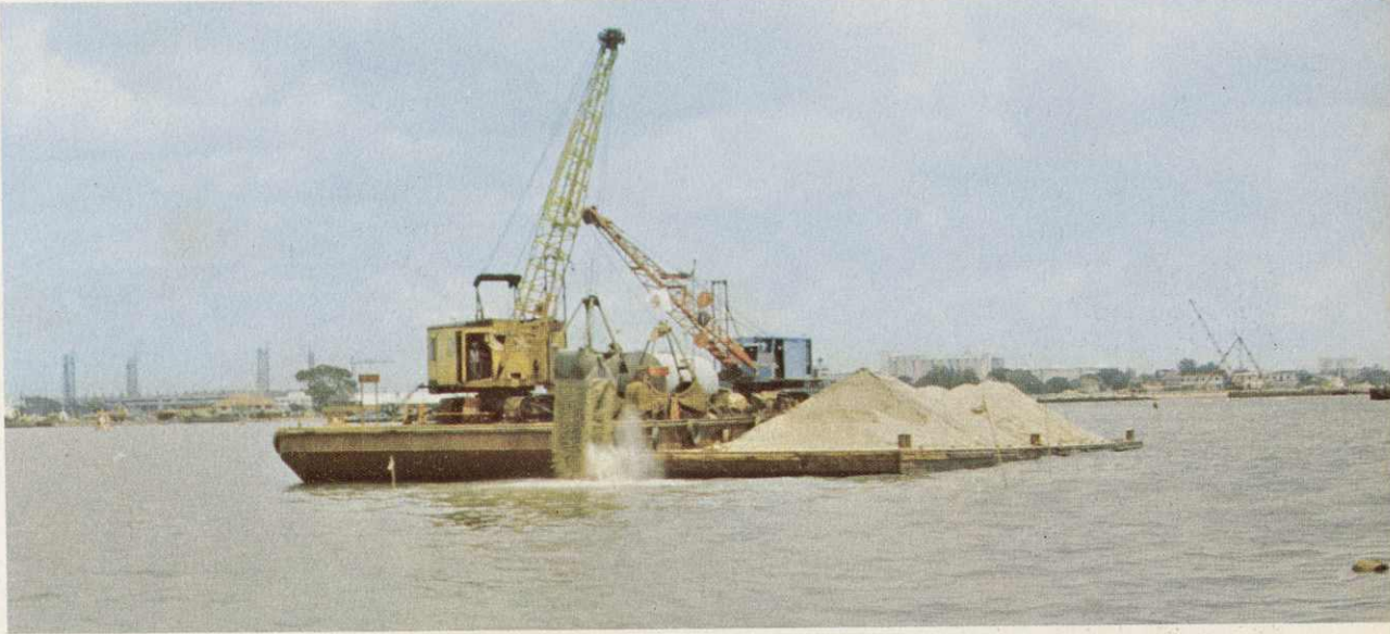
Sand-filling of dredged channel for stabilisation of sea-bed in the East Coast Reclamation, Phase III.
