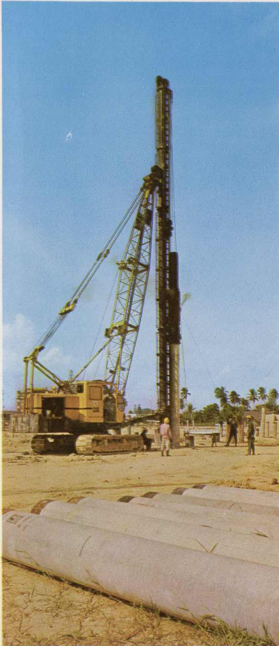
Housing Board's own piling plant in operation. The Board has set up a piling plant for the manufacture and driving of concrete piles. About 30% of the piling works for public housing are executed by the Board's own piling plant.
