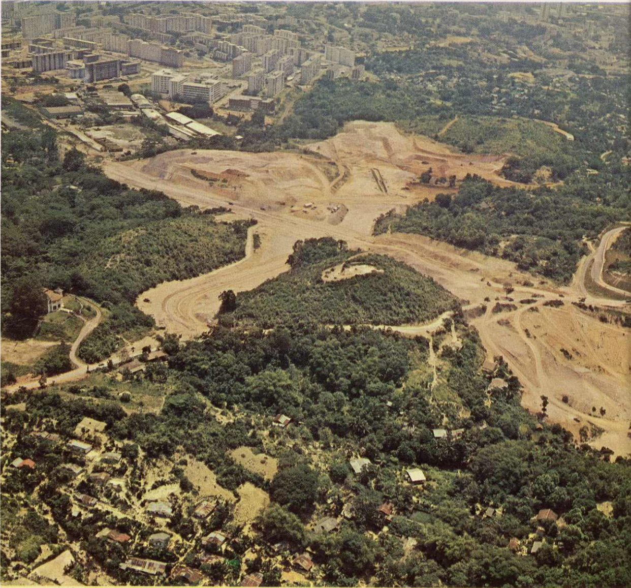
An aerial view showing the commencement of construction work in Telok Blangah New Town. In the foreground are squatter huts which are in the process of being cleared. The background shows public housing in Tiong Bahru area.
