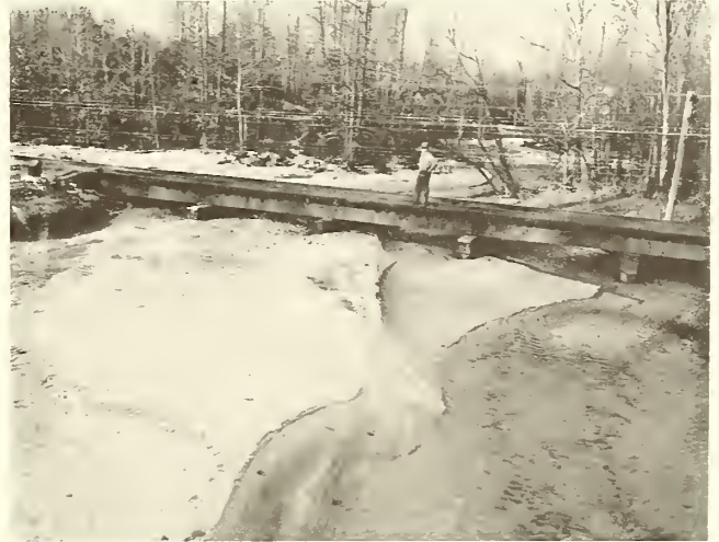
Figure 3.—This railroad bridge had to be raised three times at a cost of $300,000 because sand eroding from the hillsides repeatedly choked the stream channel.
