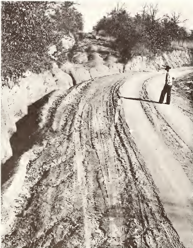
Figure 7.—Roadbank erosion accounts for 12 percent of the sedimentation on the Y-LT Flood Prevention Project.
