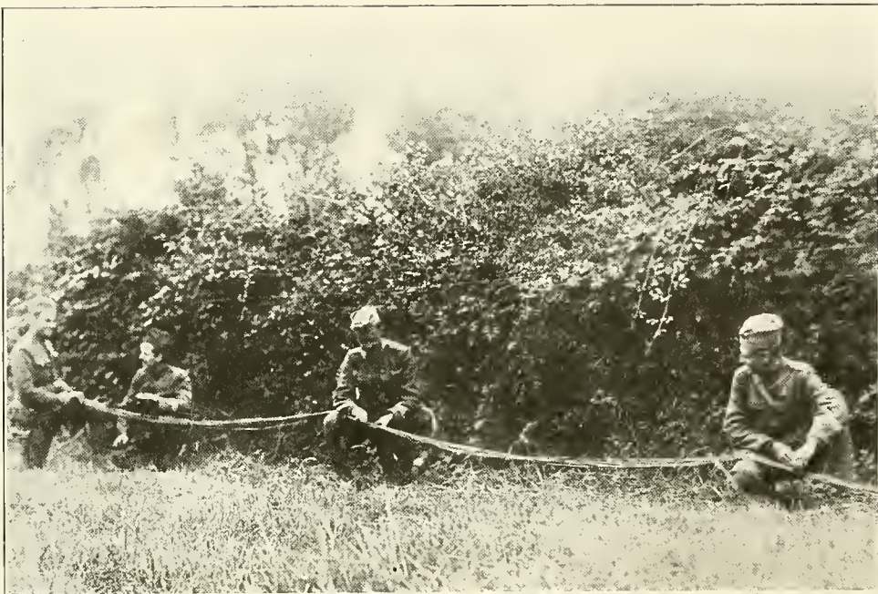
A DETACHMENT OF THE 102 ND FIELD SIGNAL BATTALION Laying a cable in the advanced area at St.-Laurent.
