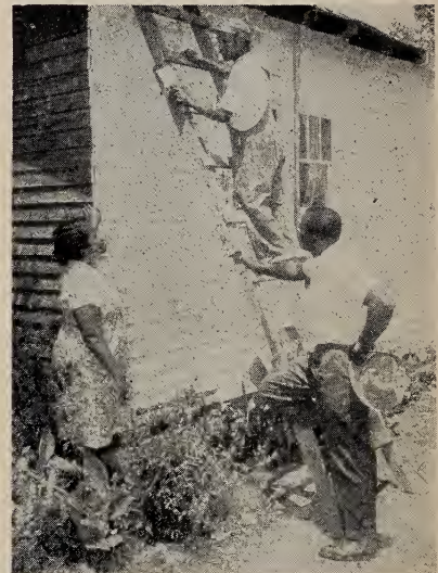
Joining in the communitywide improvement project, Mrs. Joe S. Harris is having her home painted. Talking to the painter are Mrs. Harris and County Agent Percy L. White. Twenty-seven homes in the Leeds community (Ala.) have been painted since the drive was launched.
