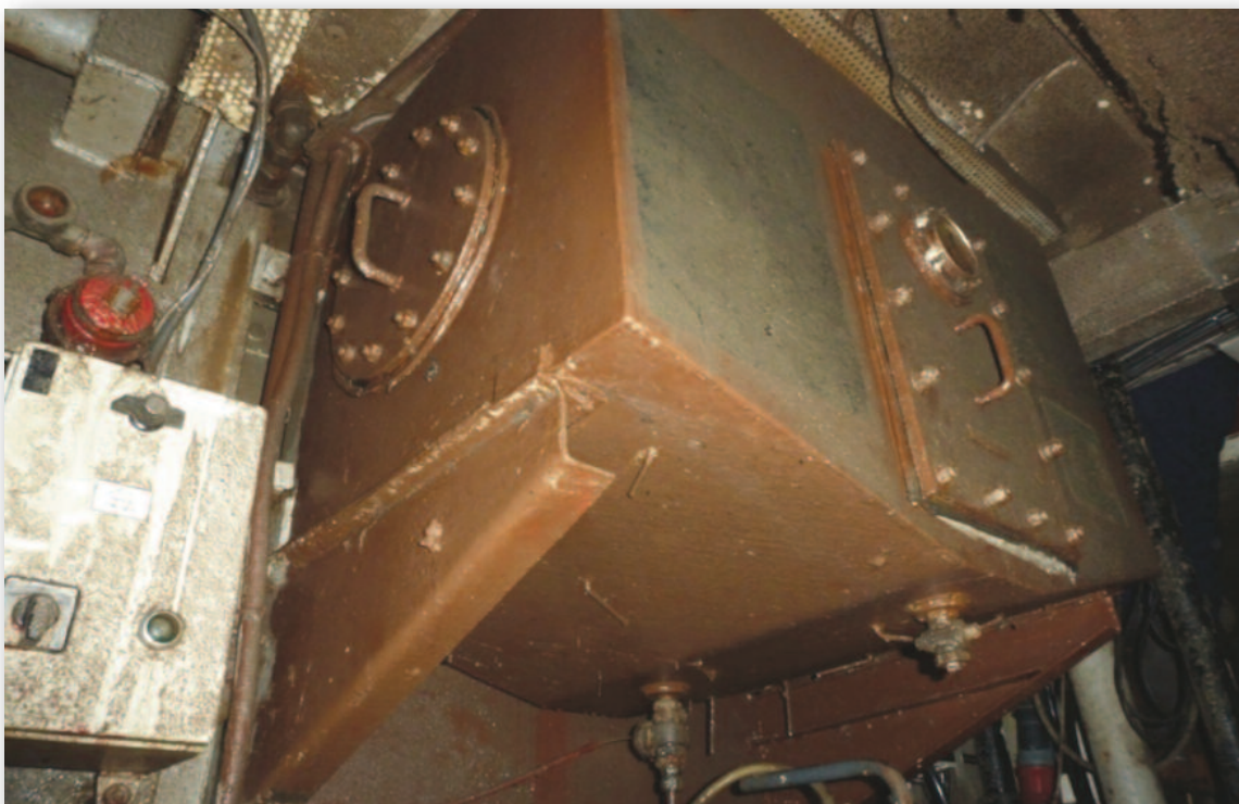
Photograph No.16 - Fuel oil daily service tank full of seawater as expected
