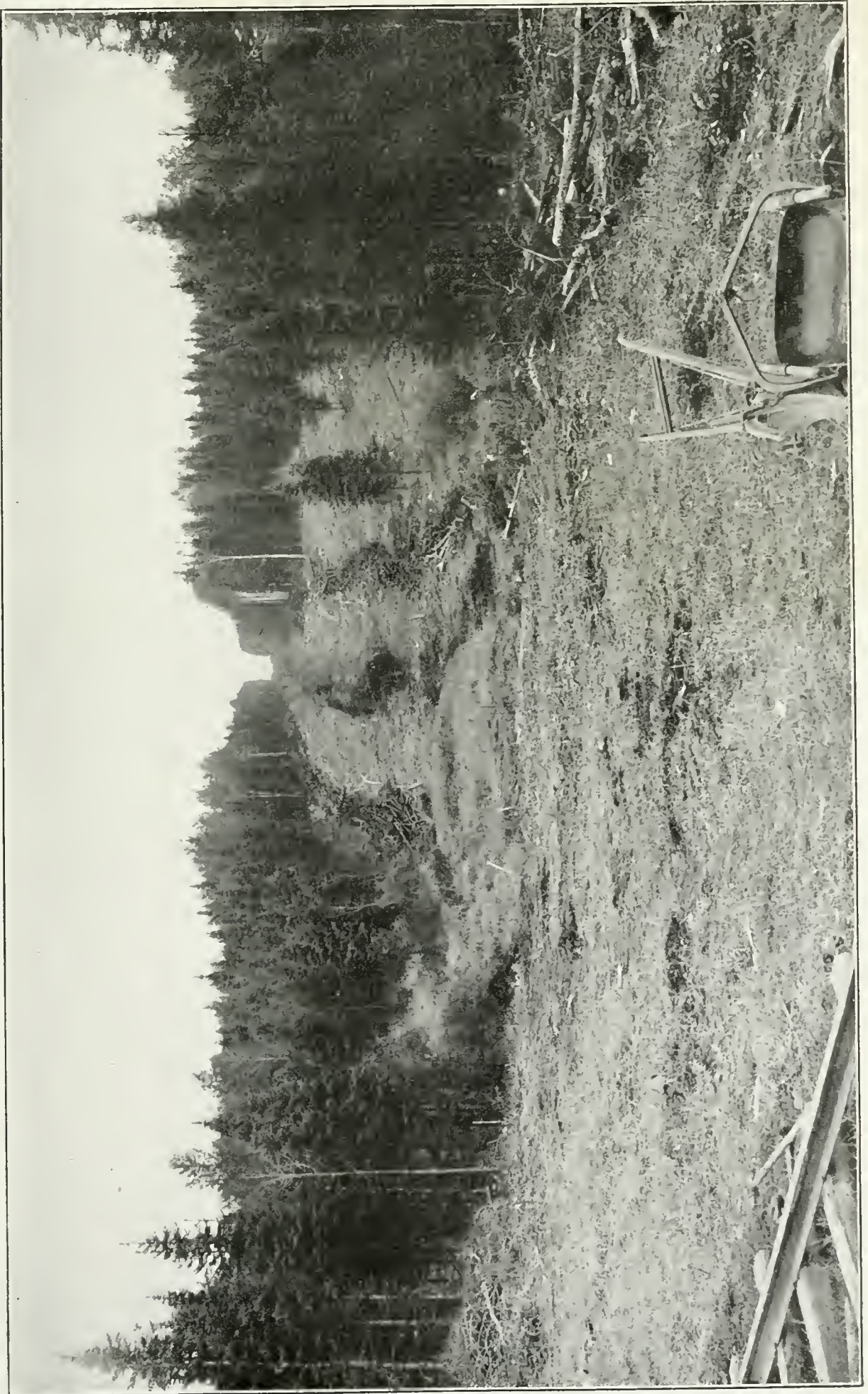
Cutting out a trunk road east from the town of Cochrane to the Abitibi River.
