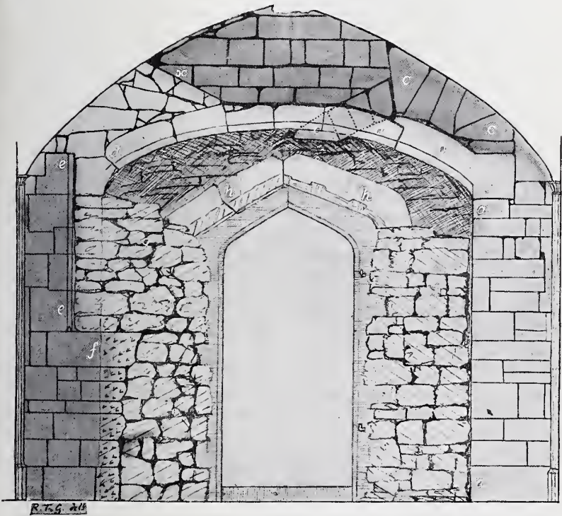
MAGDALEN COLLEGE, OXFORD. WEST WALL OF CHAPEL PORCH AFTER REMOVAL OF PLASTER IN 1901.
