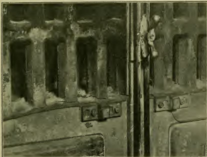
CRACKED SECTION IN BOILER RATED AT 16,800 SQUARE FEET. BOILER WAS RED HOT WHEN OIL BURNER WAS SHUT OFF.
