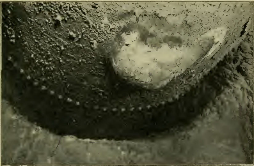
BAGGED BOILER SHELL RESULT OF SCALE DEPOSIT.
