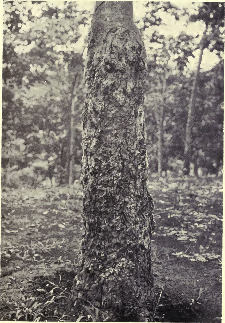
FIG. 36.—An Old Tree overgrown with Burrs as the result of Bad Tapping.
