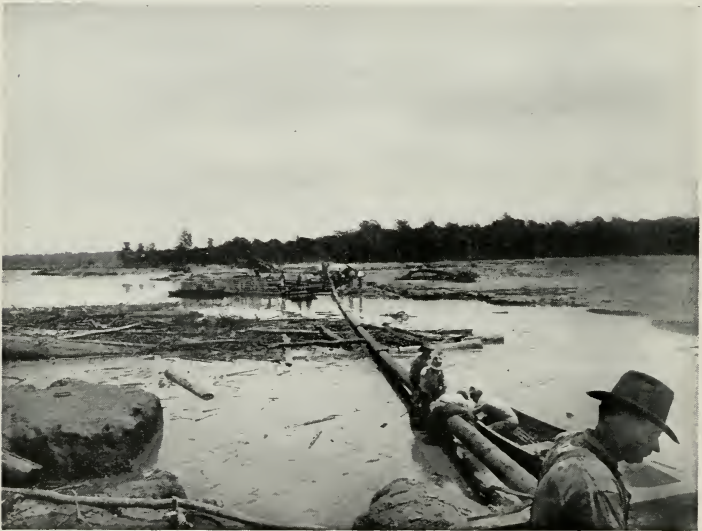
Fig. 101—Laying Temporary Line across the Red River (Ark.) In midstream Line was Floated on a Log Raft. The Water was 25 Feet Deep at that Point
