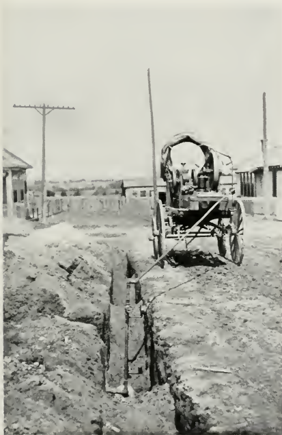
Fig. 170—TESTING A SECTION OF LOW PRESSURE SYSTEM WITH A SMALL AIR COMPRESSOR AND GAS ENGINE FOR POWER INSTALLED ON A WAGON
