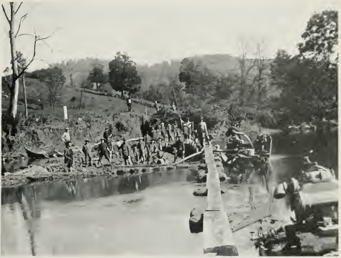
Fig. 77—LAYING 12" HIGH PRESSURE LINE ACROSS TYGARTS VALLEY RIVER, NEAR BELINGTON, WEST VIRGINIA
