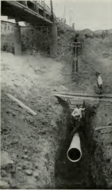
Fig. 79—HIGH PRESSURE GAS LINE ACROSS TRINITY RIVER NEAR DALLAS, TEXAS.
