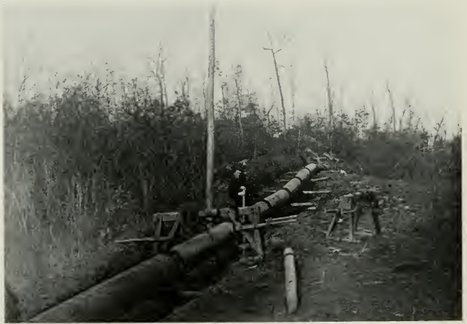
Fig. 92—PLAIN END PIPE LINE COMPLETED Ready to lower into ditch by use of wooden horses and snubbing rope.
