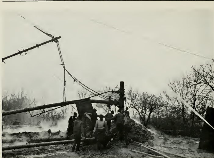
Fig. 30—PUTTING OUT A BURNING WELL IN THE CANEY FIFLD BY USE OF A HOOD AND LEAD LINE TO CARRY GAS TO ONE SIDE FROM WELL
