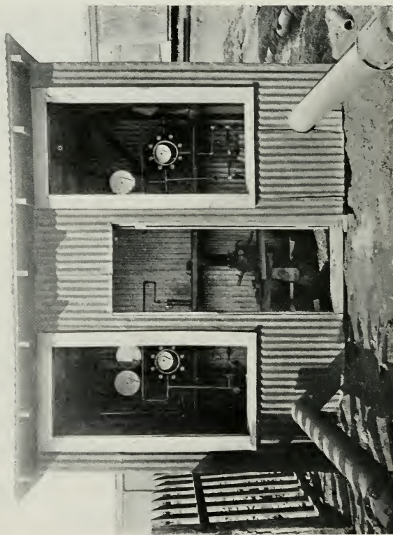
Fig. 133—INSTALLATION OF TWO ENCASED TYPE OF ORIFICE METERS
