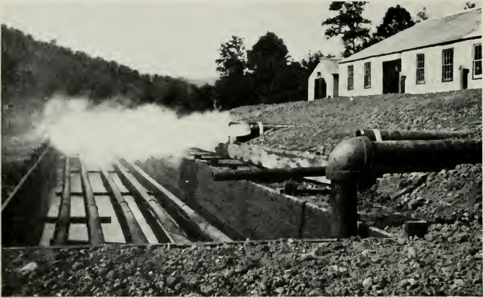
Fig. 119—EXTERIOR VIEW—GAS COMPRESSING STATION Jefferson County Gas Company, Loleta, Pa. Note Cooling Tank. The pipes in the cooler are covered with water during operation.
