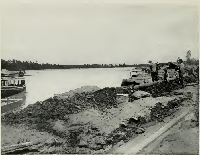
Fig. 100—Laying Temporary Pipe Line across Red River (Ark.), showing where Line leaves the new river bed
