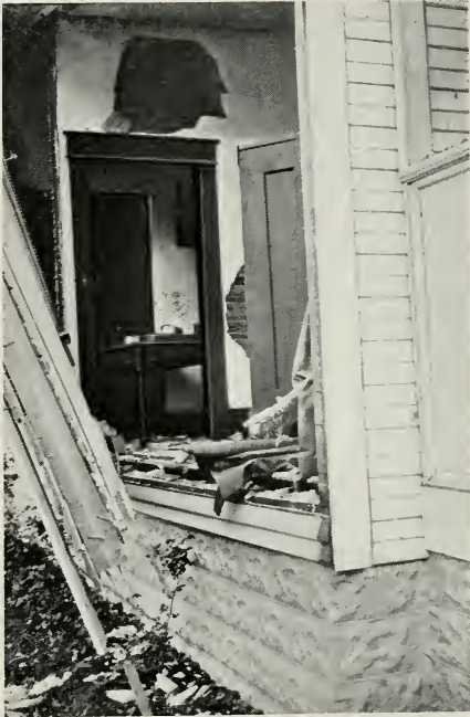
Fig. 207—AN EXPLOSION OF NATURAL GAS IN A PRIVATE HOME INDIRECTLY DUE TO USING RUBBER TUBING FOR STOVE CONNECTIONS
