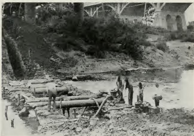
Fig. 82—HIGH PRESSURE GAS LINE ACROSS THE TRINITY RIVER Near Dallas, Texas. Note the small gasoline engine and pump for keeping water out of ditch while line is being laid.
