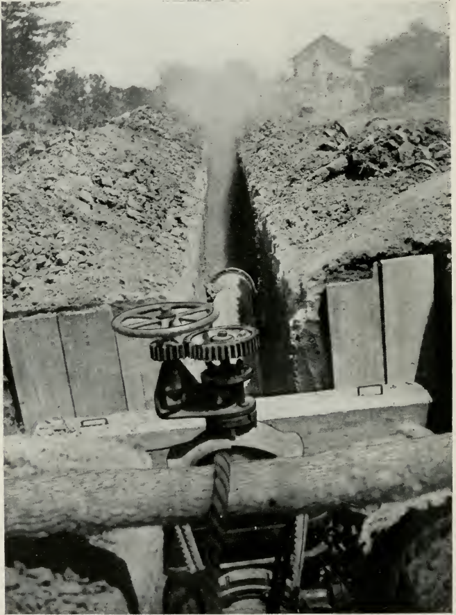
Fig. 98—BLOWING OUT 16-INCH GAS LINE BEFORE PLACING IN USE Note the Anchorage or "Deadmen" to Prevent Line Pulling Apart on Account of Pressure on Line Before Completion.
