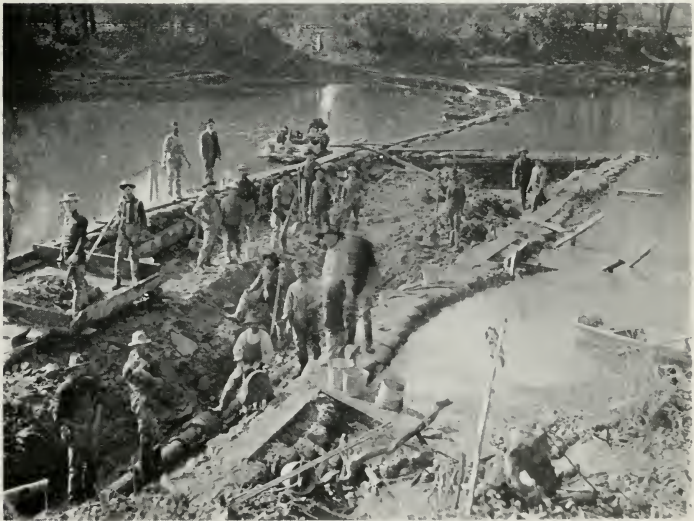
Fig. 78—LAYING 12" HIGH PRESSURE LINE ACROSS A RIVER SHOWING COFFER DAM TO KEEP OUT WATER WHILE LINE IS LAID IN CONCRETE
