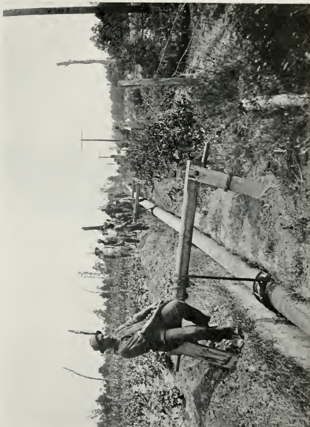
Fig. 93—LOWERING COMPLETED PLAIN END PIPE LINE INTO THE DITCH BY USE OF WOODEN HORSES AND A SNUBBING ROPE
