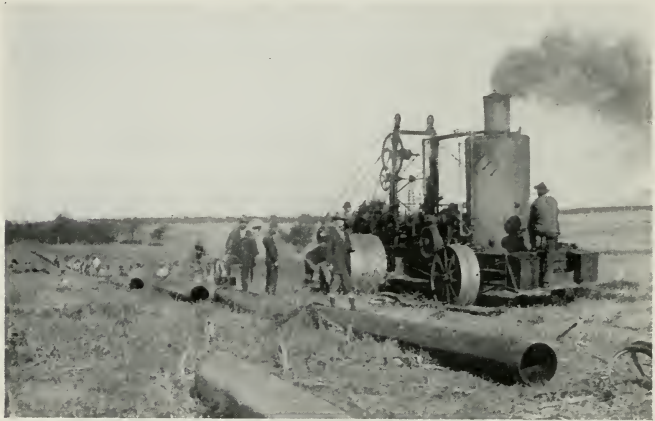
Fig. 66—DITCHING MACHINE AT WORK FOR A 16-INCH LINE Between Petrolia and Dallas, Texas, for the Lone Star Gas Company
