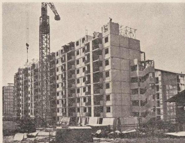
Erection of pre-fabricated flats at MacPherson Road (South) Estate under an experimental scheme.
