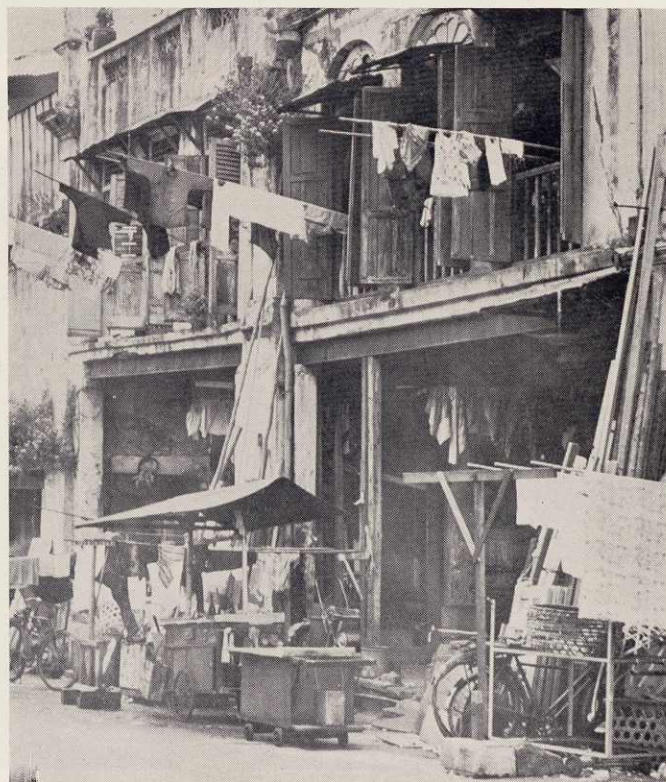
A close-up of a typical slum building in Precinct S1. Structural beams have sagged and are temporarily propped up by occupants.
