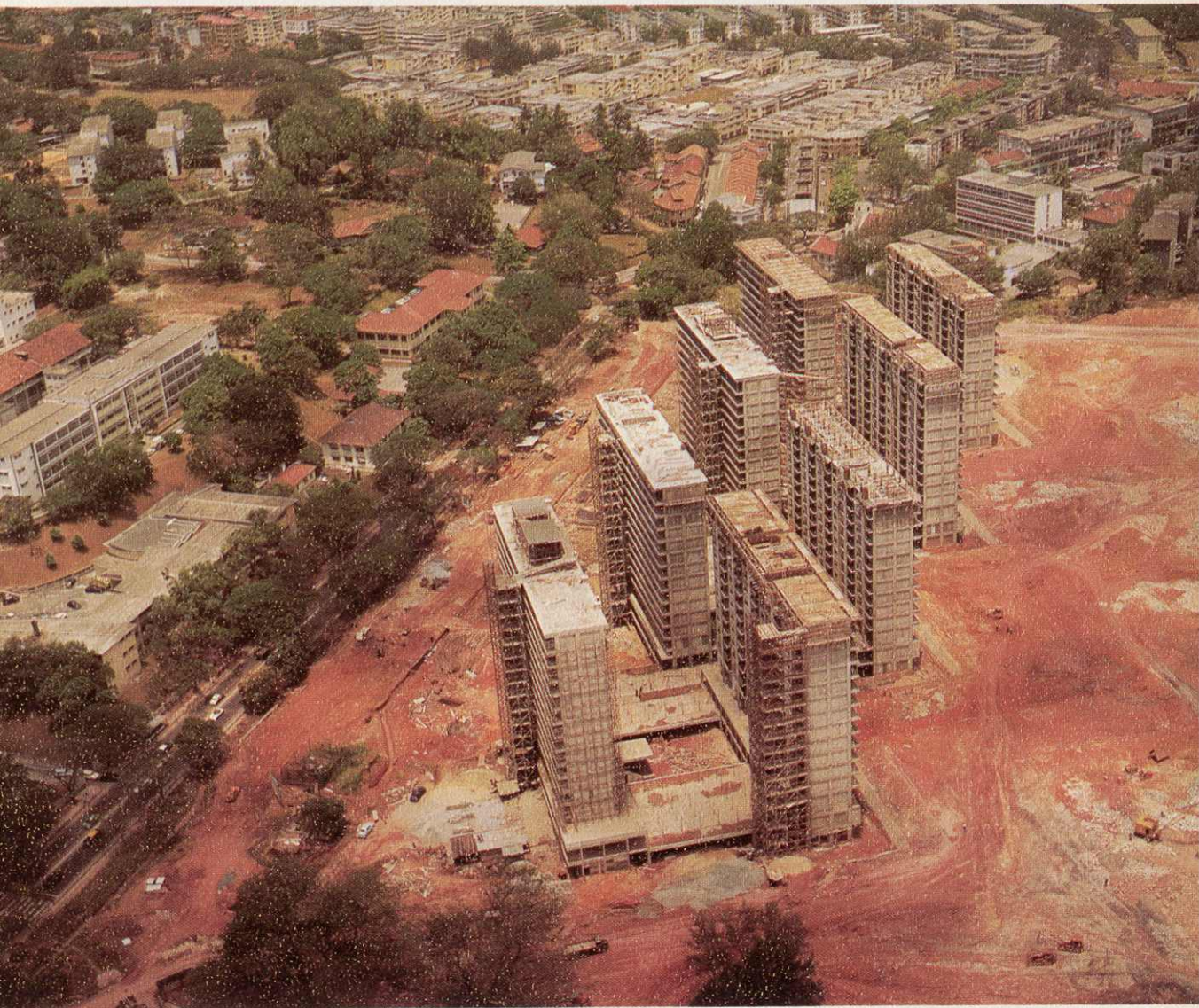
Aerial view of Precinct South 1, Contract III. Outram Road Redevelopment under construction.
