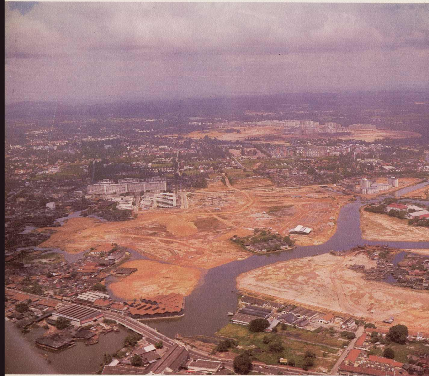
Aerial view of Kallang Basin Reclamation Scheme showing newly-reclaimed land and the two flatted factories in background. 400 acres of swampland are to be reclaimed from the Kallang Basin for labour intensive industries and low cost housing.
