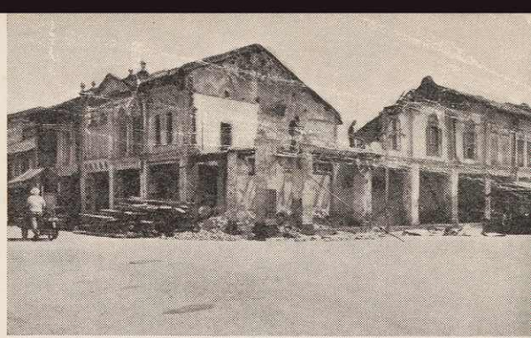
Obsolete buildings in Precinct N1 being demolished under the Board's urban renewal programme.
