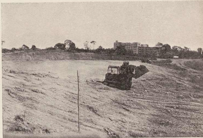
A site at Toa Payoh which has been cleared of squatters and is being levelled for construction purposes.
