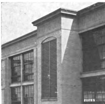
Air is drawn in through ventilators at the top of the building where the air is purest
