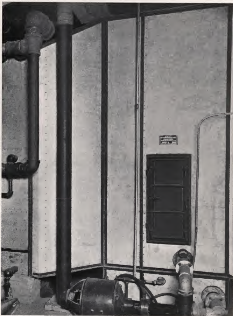
CARRIER TYPE C WASHER INSTALLED IN NATIONAL THEATRE, DETROIT, MICH.
