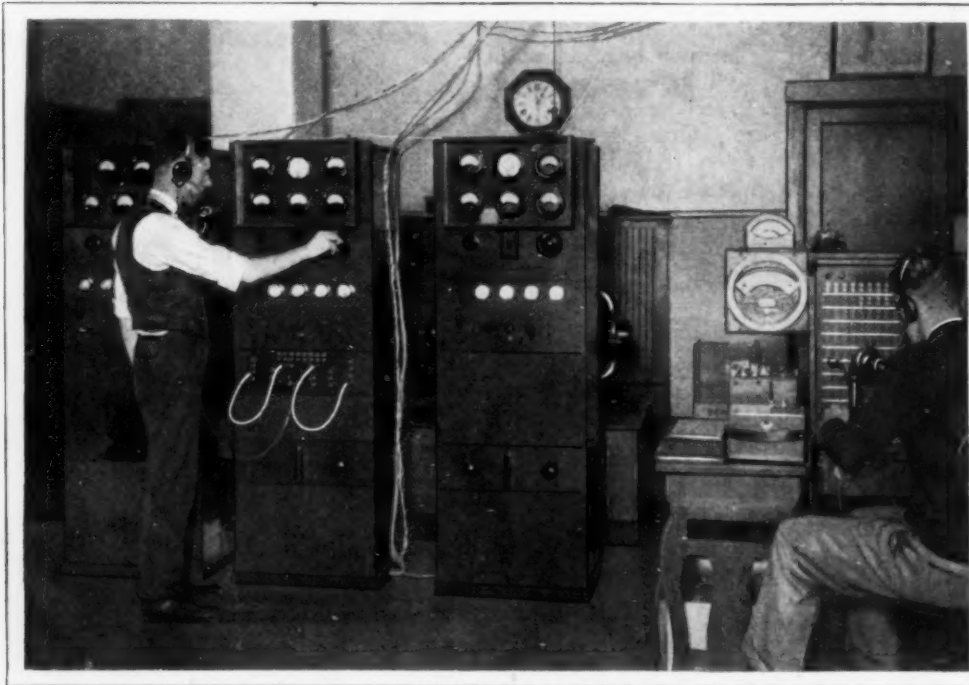
Three Radio Transmitters, for Three Different Wave Channels, Installed in the Telephone Office at Freeport, Ill.; the Wires Leading Out at Top Connect with the Phone Cables
