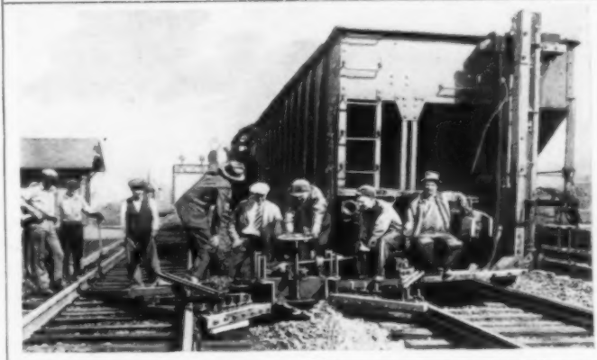
Ballast Spreader Devised by Foreman of the Pennsylvania Railroad; It Is Based on Principle of Farm Harrow
