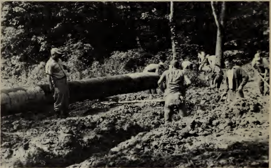
The Silver Trail, a road to the Kentucky Woodlands Refuge Headquarters, was reditched and regaveled under the accelerated public works program to provide access to a visitor center to be constructed on the refuge.
