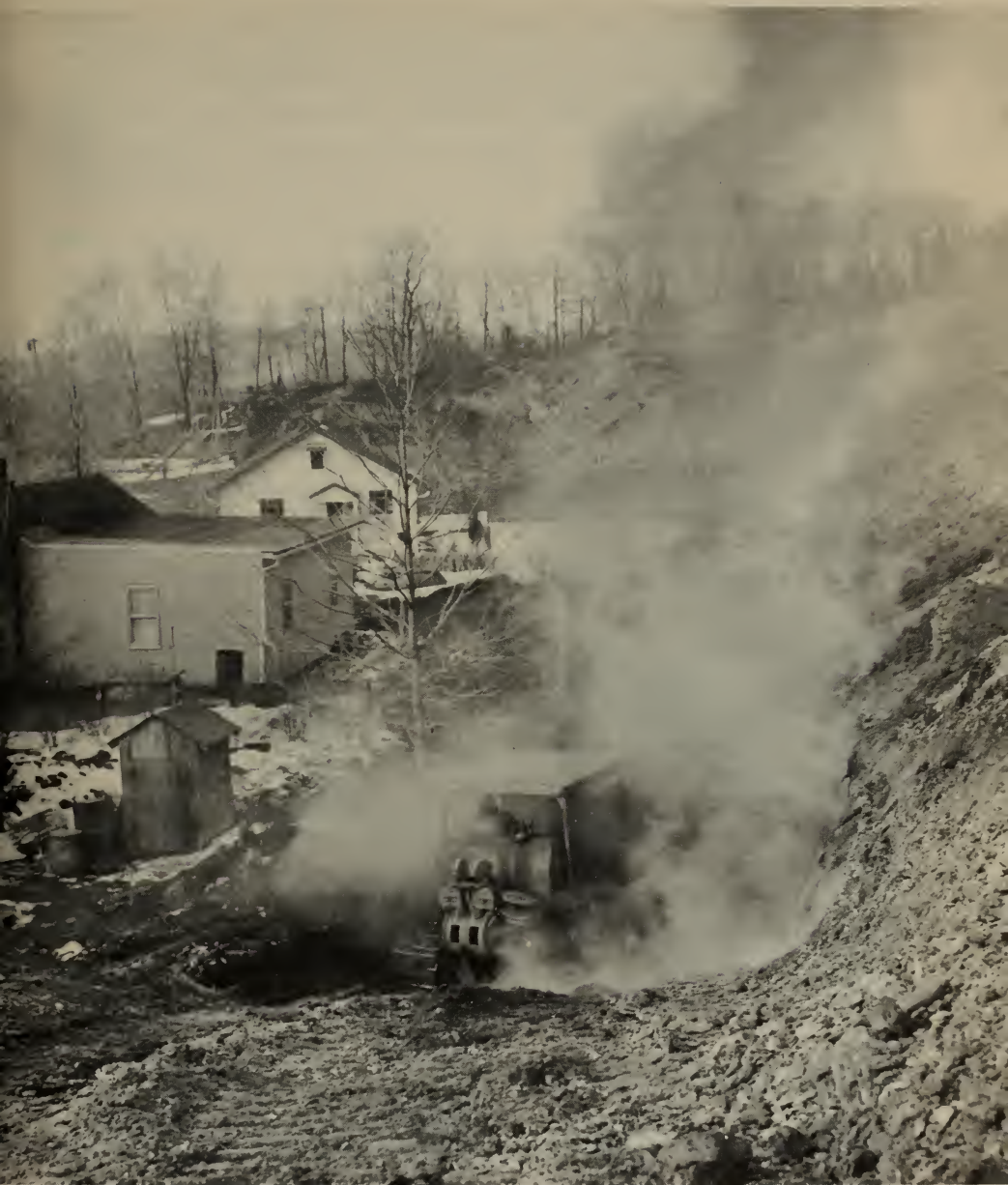
Under the direction of the Bureau of Mines, a protective trench is being dug between these Pennsylvania homes and a fire in an abandoned coal mine. More than 30 such projects have been carried out in recent years under a cooperative agreement between the Department and the Commonwealth of Pennsylvania.
