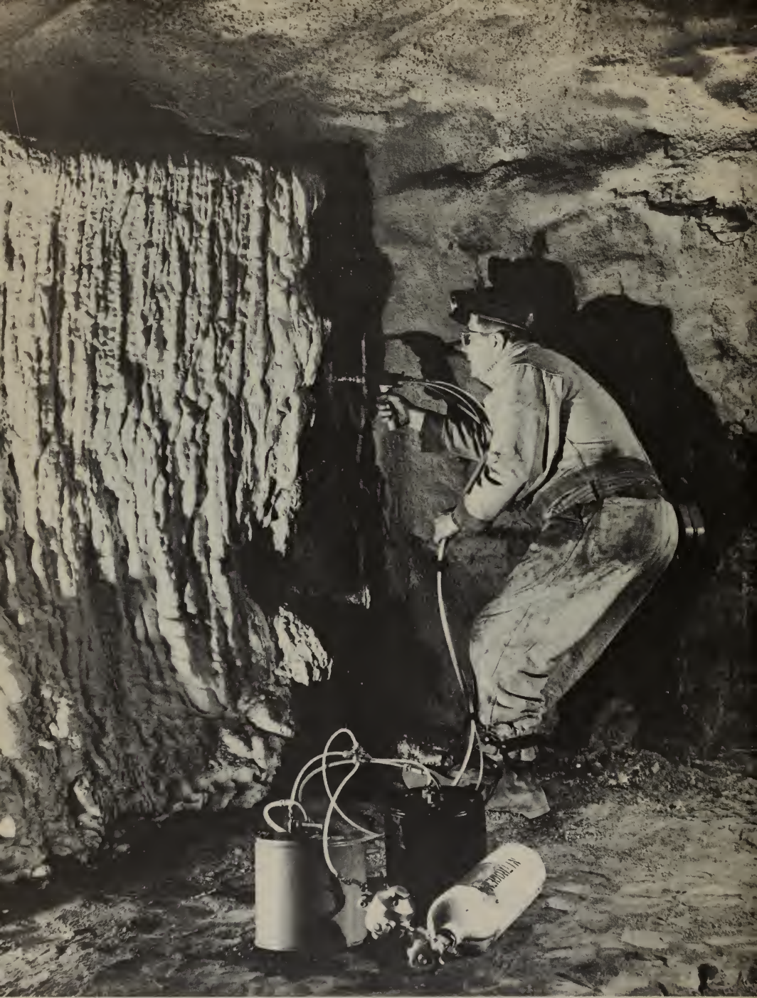
A Bureau of Mines technician uses portable equipment to block off a mine passage with waterproof, fire-resistant rigid foam. Developed by the Bureau last year, the plastic foam has recently proved its usefulness in such applications as mine-water control and firefighting.
