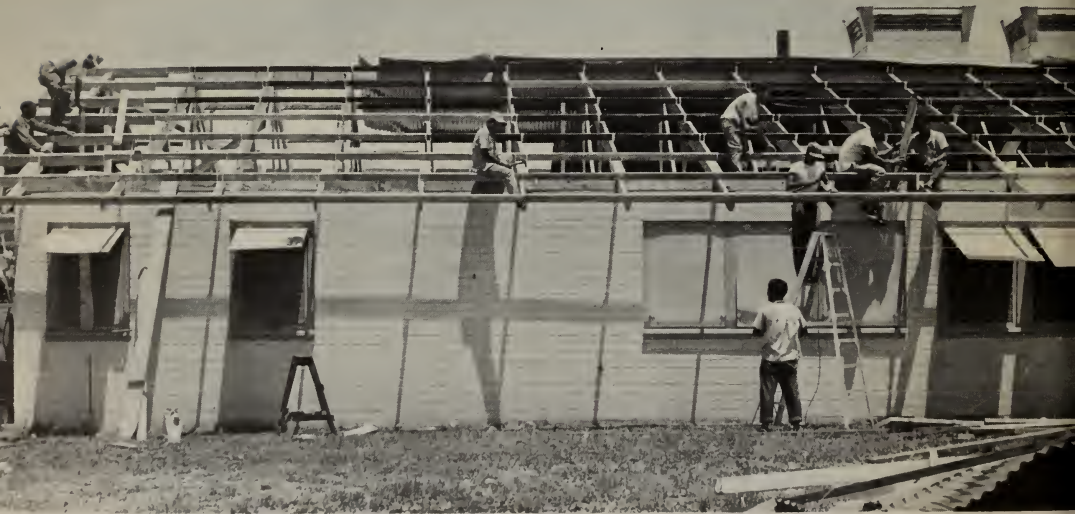
Public works crew is shown replacing the roof of Torres Memorial Hospital in Saipan after Typhoon Olive unroofed the hospital buildings.
