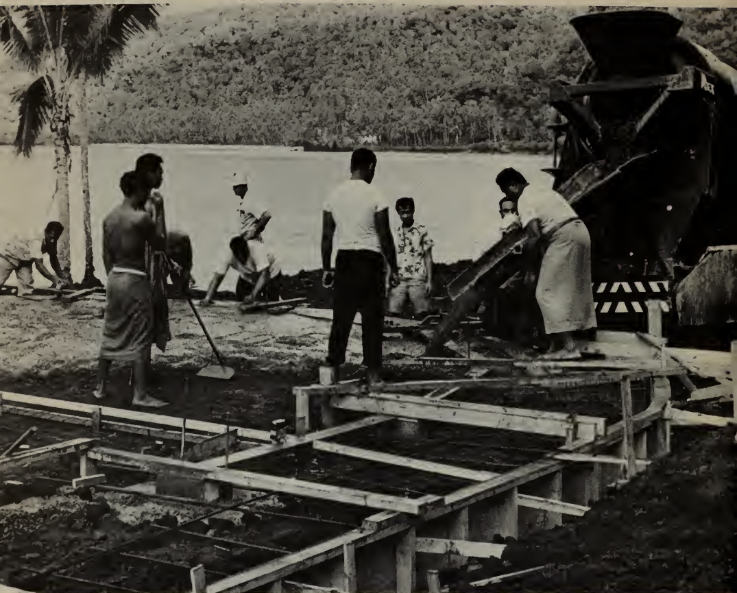
Samoaans employed by accelerated public works poured the first concrete in May 1963 in constructing for the educational television consolidated elementary school program at Nua Village on American Samoa's main island of Tutuila.
