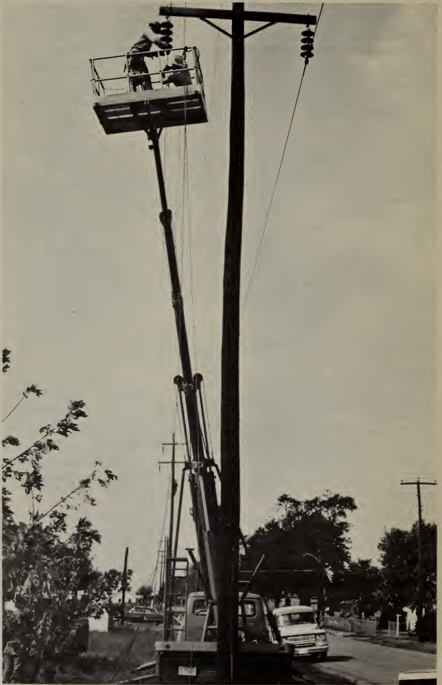
Southwestern Power Administration's "snorkel" truck is an example of efficient application of the machine for greater manpower utilization.
