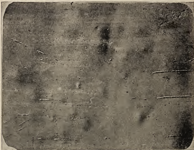
FIG. 49.— Appearance of the exposed surface of corroded tinned copper sheathing used for roofing purposes. \times 1
