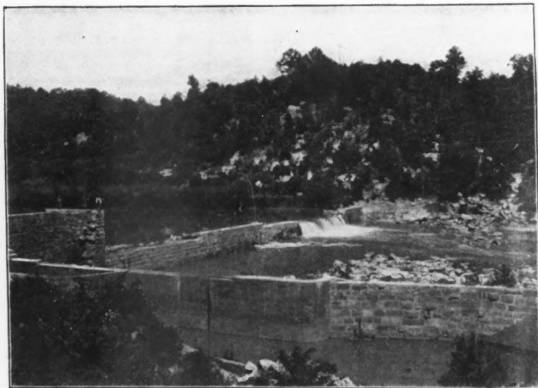
FIG. 1. PEDLAR DAM, ON THE JAMES RIVER, BEFORE REPAIRS WERE MADE.
