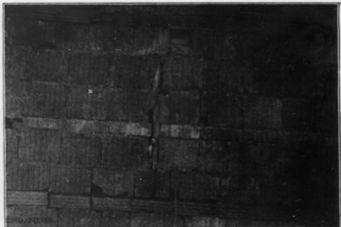
FIG. 3.—SHOWING BADLY BROKEN TILE, DISCONTINUOUS RINGS, ECCENTRIC KEYS, HOLES FILLED WITH SPALLS, ETC.
