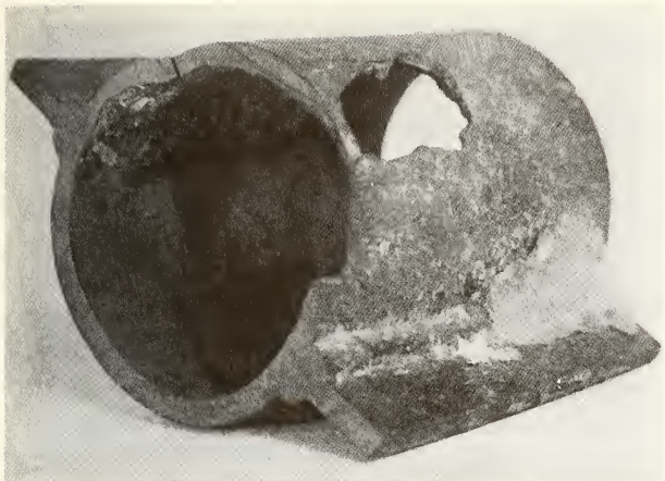
Fig. 1. Cut length of a high-pressure boiler tube corroded from the inside (the waterside), showing thick-edged hole about 4 cm long where steel embrittled by hydrogen (corrosion by-product) was violently ejected while boiler was operating.
