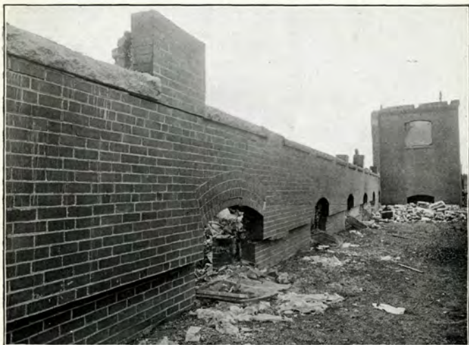
West Wall, No. 6 Weave Building, as pushed out by expansion of steel floor beams.
