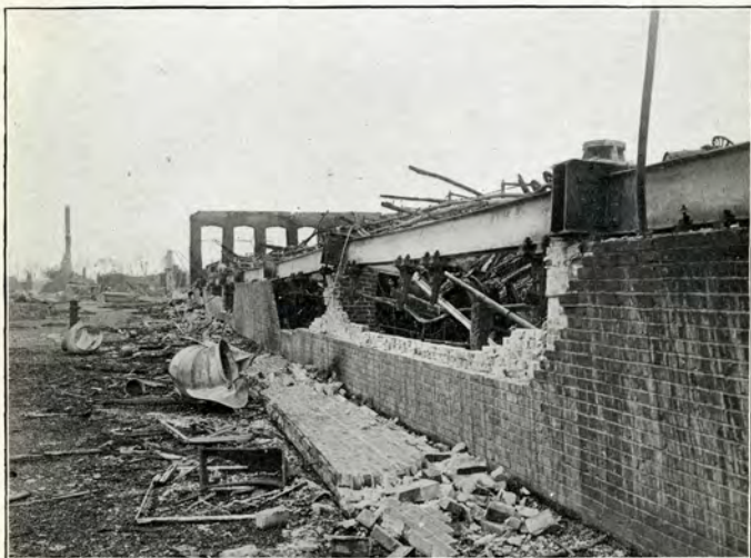
South Wall, No. 6 Weave Building, thrown over by expansion of steel floor beams.
