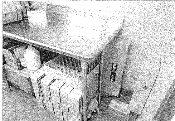
Figure 5: High Voltage Electrical Panel Installed Next to Cafeteria Dishwasher at a BIE-Operated School, October 2014
