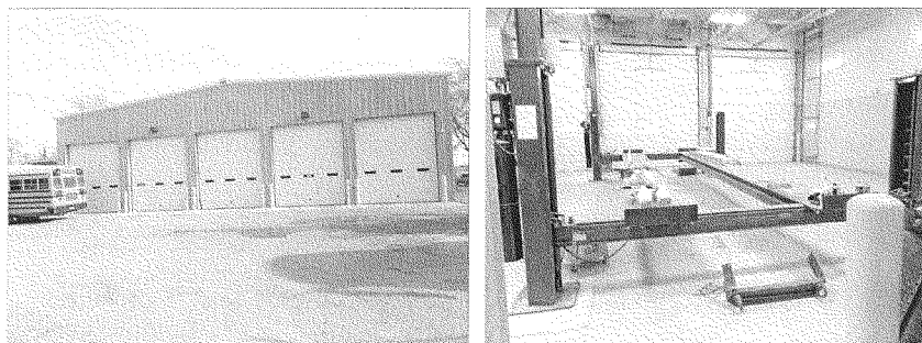
Figure 6: Exterior and Interior of Recently-Constructed Bus Maintenance Building Where Door Does Not Close When a Large School Bus Is on Hydraulic Lift
