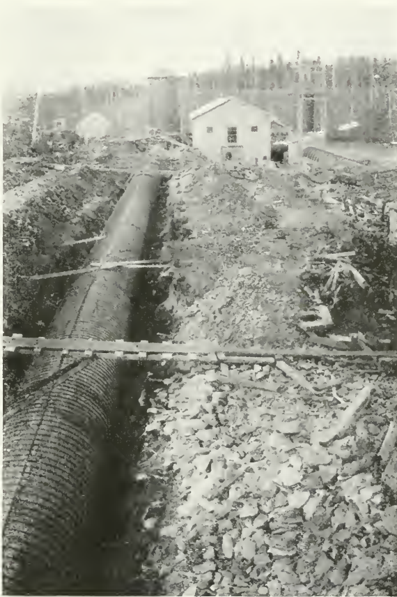
View from intake of power house showing surge tanks and wood stave penstocks at Sandy falls, Mattagami river, township of Mountjoy
