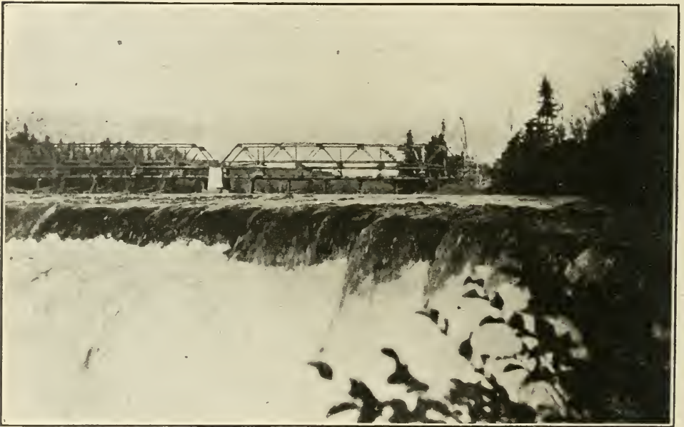
Constructing a steel bridge across the Kaministiquia River at Kakabeka Falls; 30,000 h.p. developed at this point.
