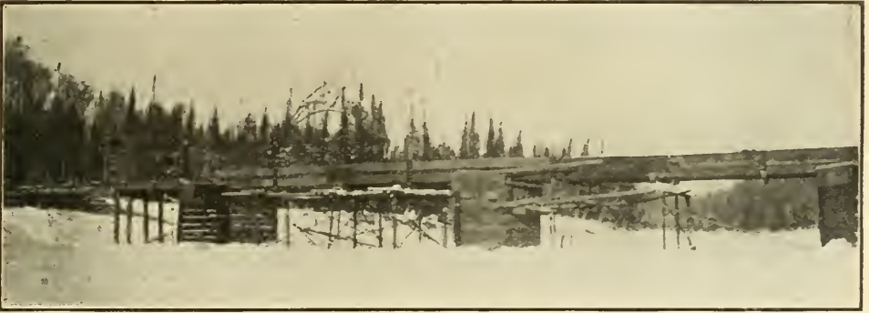
Constructing bridge at Frederickhouse River, five miles west of Cochrane; 200 ft. long.
