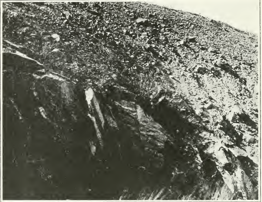
Fig. 7—Partially decomposed Keewatin rock in place near Mile 162, A.C. and H.B. Railway
