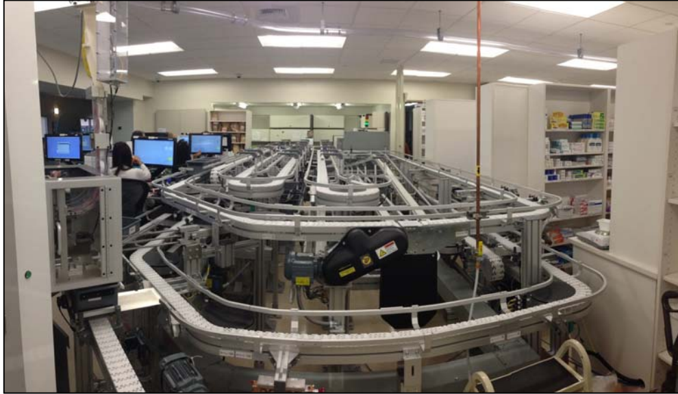
Figure 2. Conveyer Belt Installed at Naval Medical Center San Diego. Once the customer places an order, the conveyer system directs each prescription through the different steps of the fill process. Manual fill stations are located to the right side of the conveyer belt; as pharmacy technicians complete a manual fill, they place completed orders onto the conveyer belt for routing to pharmacist verification.
