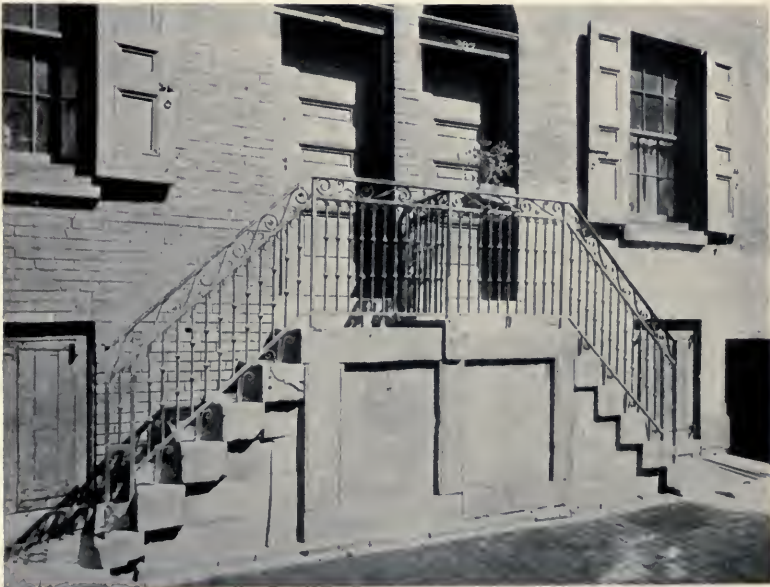
PLATE XXXVIII. — Detail of Iron Balustrade, 216 South Ninth Street; Stoop with Wing Flights, 207 La Grange Alley.
