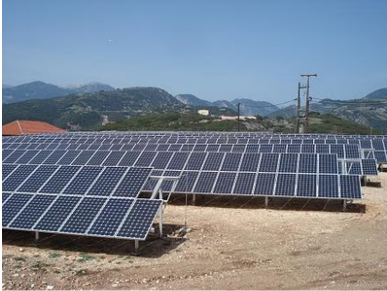
Figure 1. Photovoltaic Solar Panels
