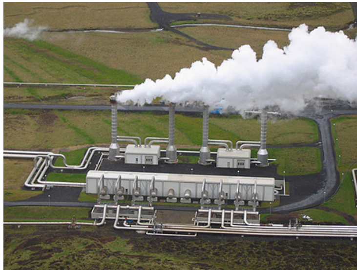
Figure 9. Geothermal Power Plant in Iceland
