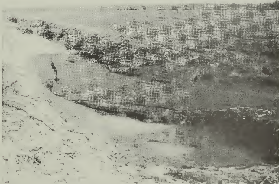
Erosion occurring from improper land management produces sediment that clogs outlet channels and drainage ditches.
