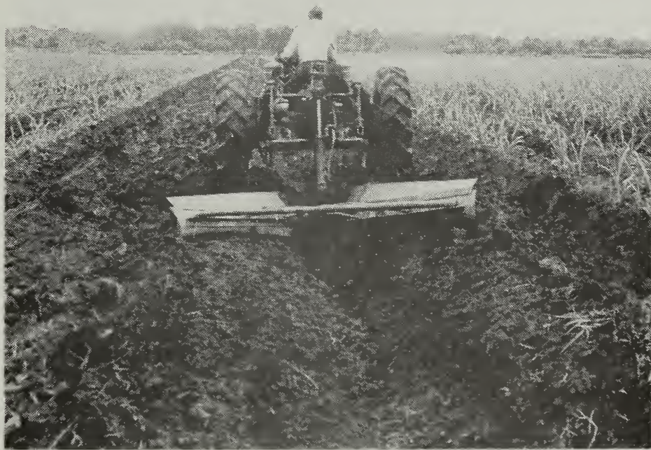
On-farm ditches are constructed to drain off excess water and convey it to outlet channels.
