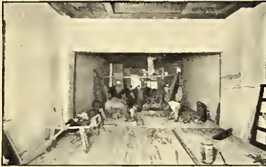
Construction work was recently carried out to connect the Barclay Street and Vesey Street Stores of the Stumpp & Walter Co., the combination making an exceptionally large area for the display of merchandise and the prompt attention to purchasers.
