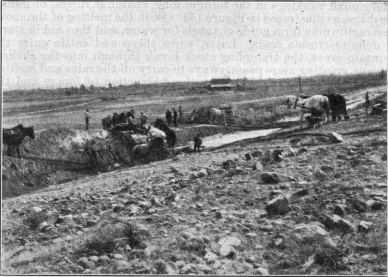
FIGURE 156.—Expensive break in irrigation ditch near Kennewick, Wash., caused by water finding its way through burrows made by pocket gophers
