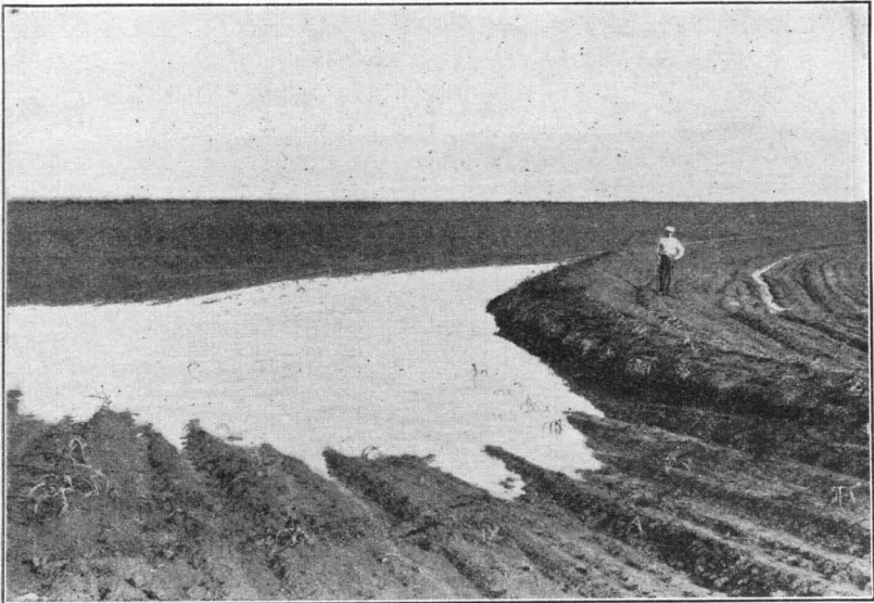
FIGURE 164.—Water impounded above terrace across a gully. Where the terrace embankment is not sufficiently wide seepage through the terrace often results in washing out terrace embankment
