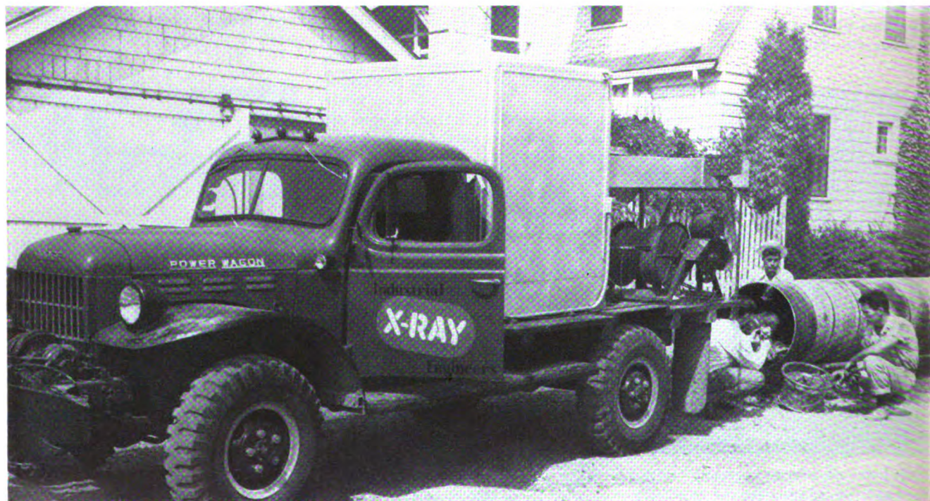
Welds in a gas pipe line are being X-rayed on the site of installation in Detroit. A complete mobile X-ray laboratory makes this on-the-spot check possible. Stray radiations from this examination are monitored by the Detroit Bureau.
