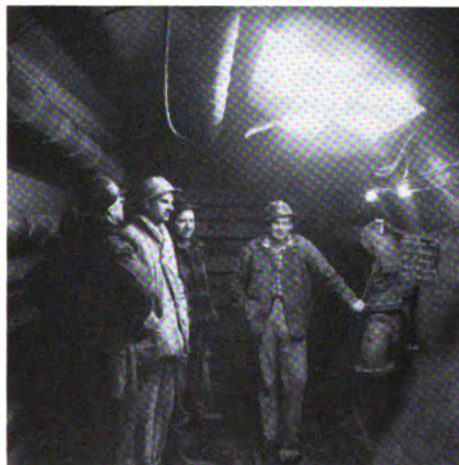
A bank of infrared lamps in the air lock is used as a source of heat during decompression.
