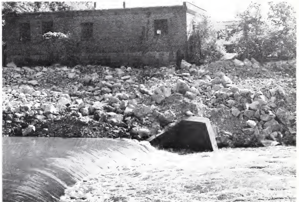
When the Waurika, Okla., water treatment plant was built many years ago, it was about 25 feet from Beaver Creek. After heavy rains last April, erosion had eaten away at the nearby banks until a corner of the plant was hanging 20 feet above the creek (top photo). Rock riprap was placed in the washed out area to stabilize the bank (bottom photo).
