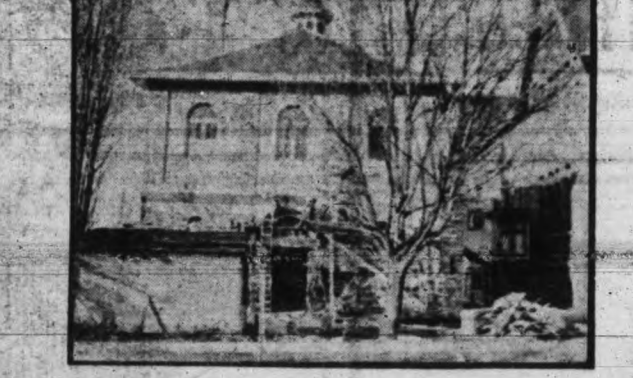
The south face of the annex for the South Park school, to provide quarters for manual training and domestic science, which is now almost finished. The building is on a lot purchased adjacent to the school, and abutting on Michigan street. A covered way connects it with the present school.
