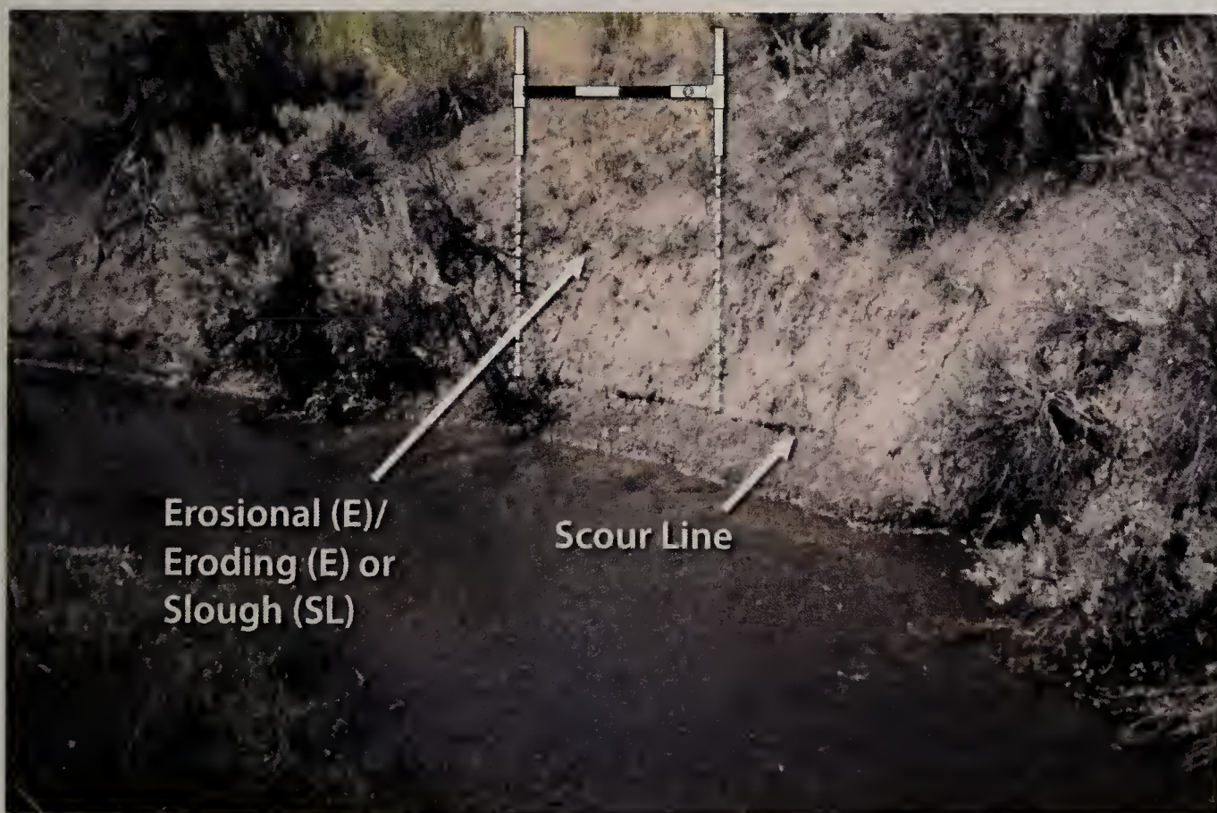
Figure 10. The streambank has an obvious scour line. The bank evaluated is above the scour line to the first bench and is recorded as erosional (E) and slough (SL) or erosional if the bank angle is within 10 degrees of vertical (Burton et al. 2011).
