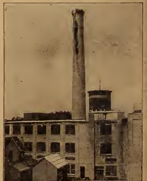
LIGHTNING'S WORK ON SMOKE-STACK
